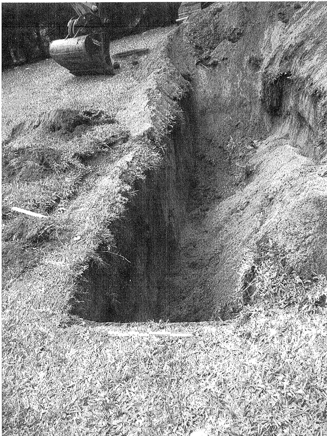
Figure 12. Trench 2 (after northern sidewall collapse), view to west.
