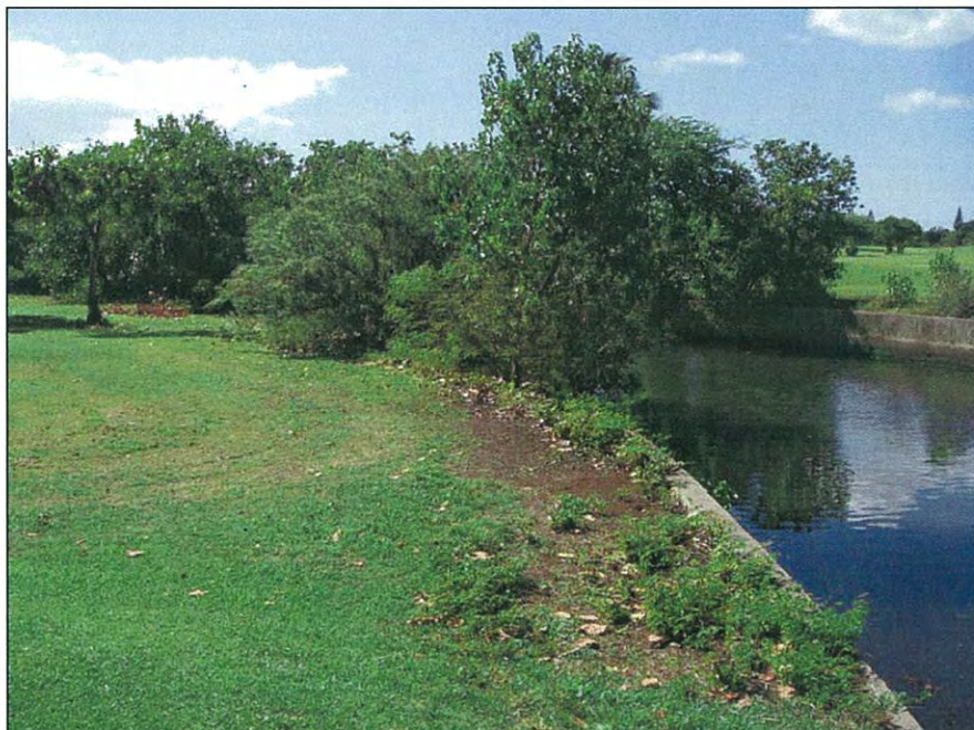
Figure 29. Photograph of drainage canal bisecting LCAs within the northwestern corner of the project area.
