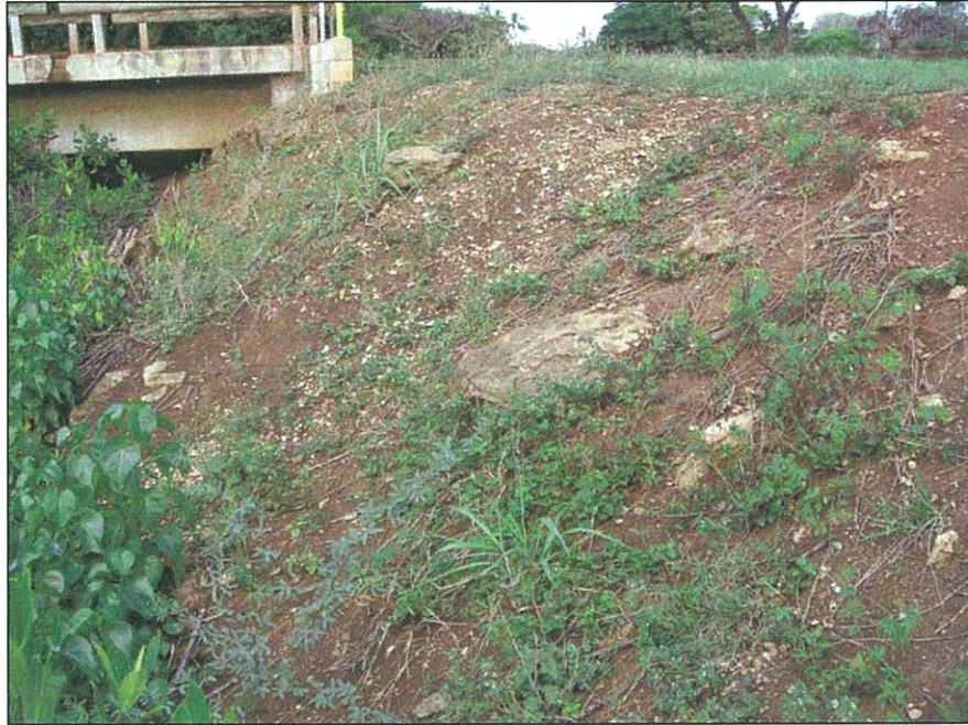
Figure 32. Photograph of exposed soil bank along drainage canal, view to west
