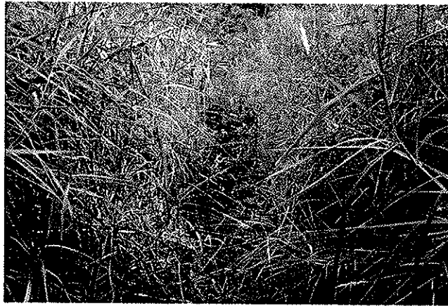
Figure 2. Slightly downward-cut stream bed upstream from the culvert on Keaau-Pahoa Road.
