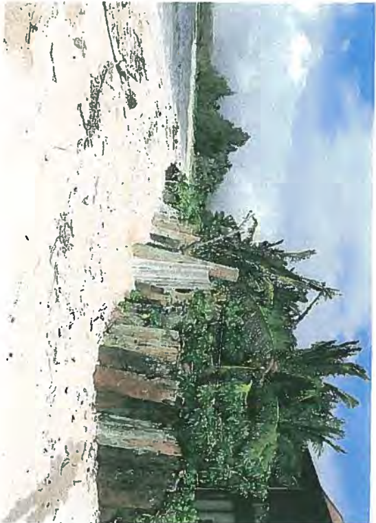
Photo 1: The pole fence on the Borsa property (Removed)
