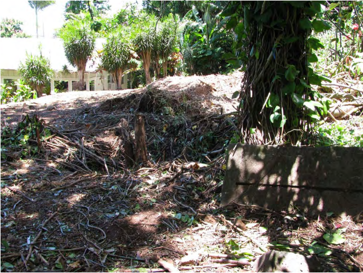
View from northwest corner of area of future construction looking southeast to edge of existing structure; ground clearing extends just beyond area of future construction;
