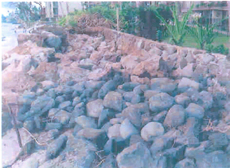
Photo showing area of 1998 repair work following completion of boulder replacement activities
