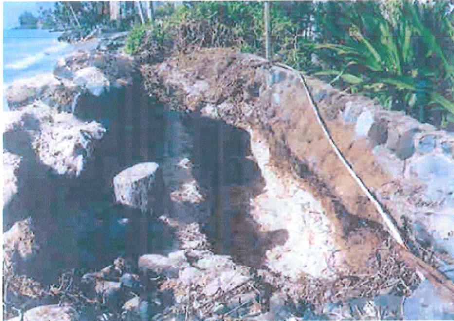
Photo showing area of 1998 repair work following completion of Naupaka removal work and trench excavation activities
