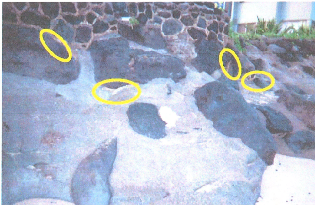
Photo showing present condition of vertical seawall and boulder revetment. The yellow circles identify areas of the existing boulder revetment (along the makai side of the vertical wall affected by the completion of the cement grouting work in 2004. It is noted that the existing boulders of the revetment were originally cemented in place during the early 1980's.
