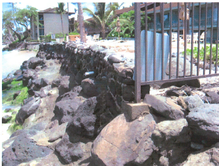
Photo showing present condition of the vertical seawall and existing boulder revetment following completion of 2004 cement grouting repair work.
