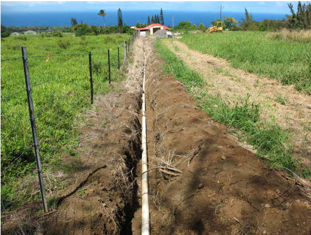
Figure 9. Open trench along the western boundary of Parcel 3-5-4-02:022, view to the northeast.
