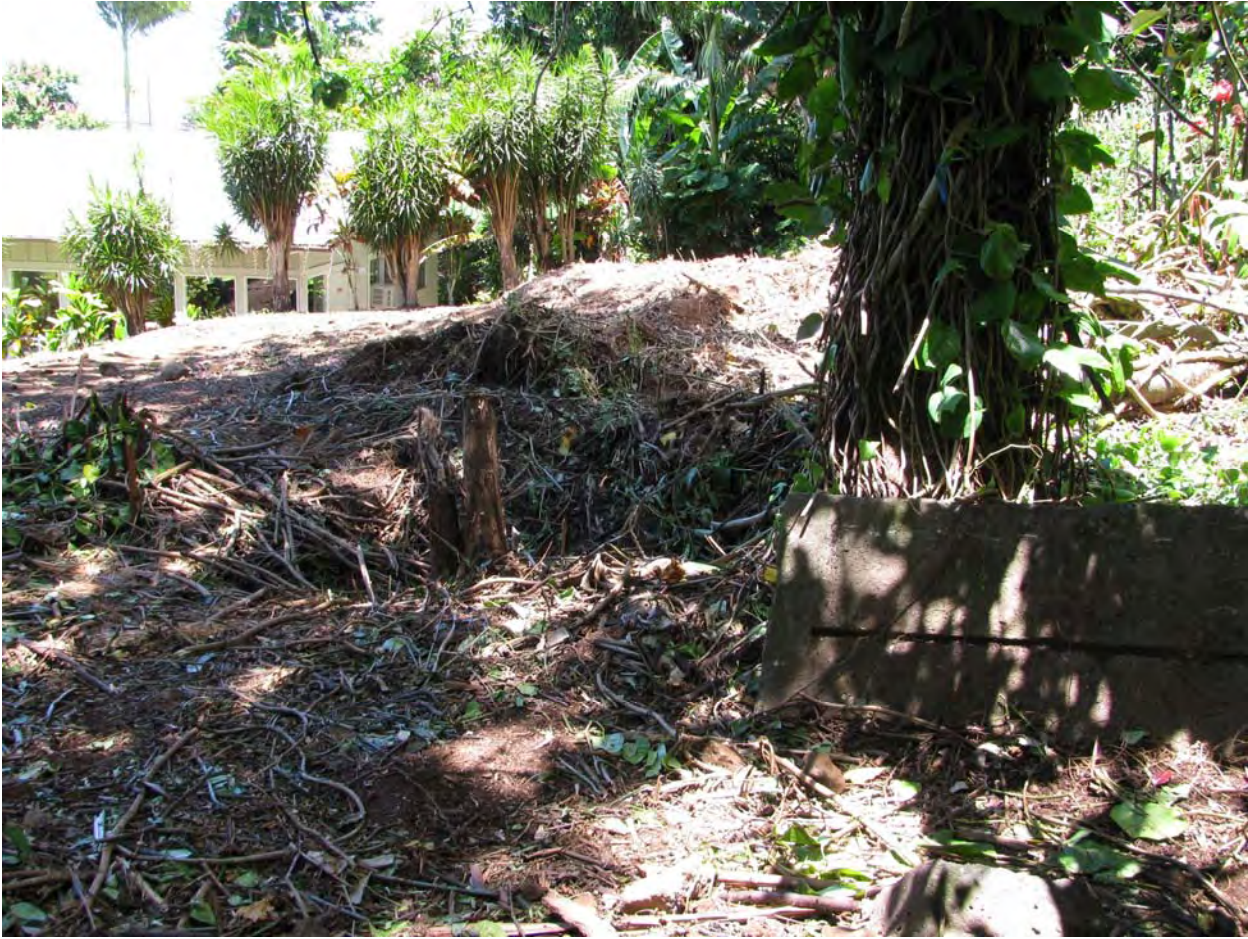
View from northwest corner of area of future construction looking southeast to edge of existing structure; ground clearing extends just beyond area of future construction; note upturned concrete floor
