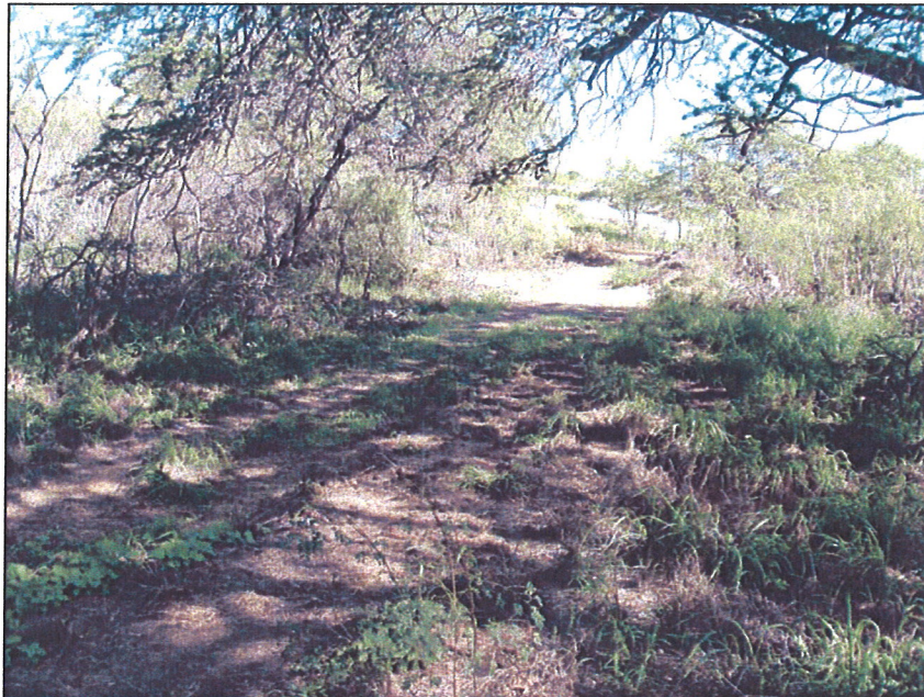
Photo # 4: Grubbed Access Road from the Edge of Baldwin High School Boundary Fence, View to Northwest.
