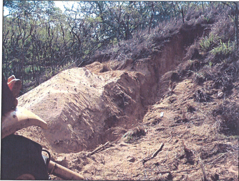
Photo # 33: BT-10 Showing Area of Collapsed Sand Slope, View to Southeast.
