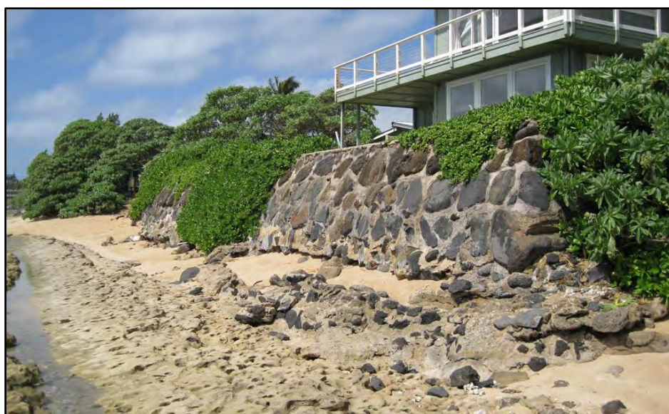
Figure 2-6 Collapsed toe and undermined seawall on neighboring property to the south
