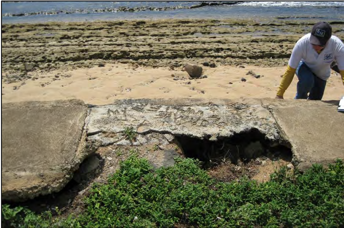
Figure 2-9 Hole in revetment cap at Station 1+05
