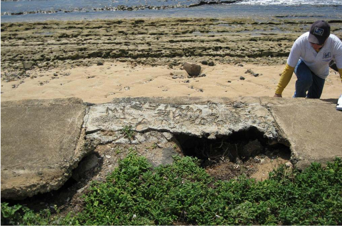
Photo 3: Erosion formed hole at station 1+05 (Source: Sea Engineering, Inc., 2011)
