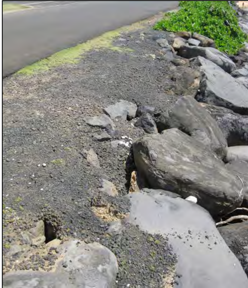
Figure 2-16 Roadway and eroding bank at Station 6+80
