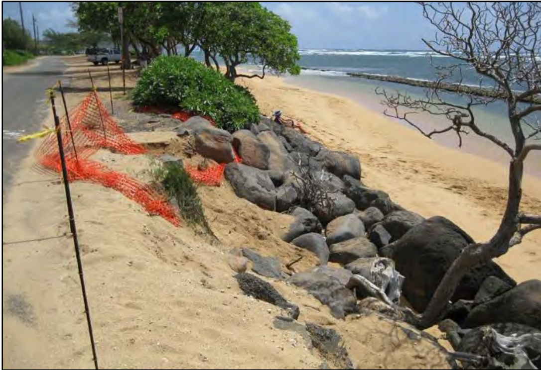
Figure 2-22 Erosion along roadway looking north from Station 9+90
