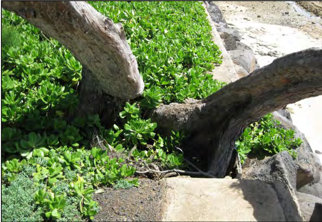
Figure 2-11 Trees and hole in revetment at Station 2+10
