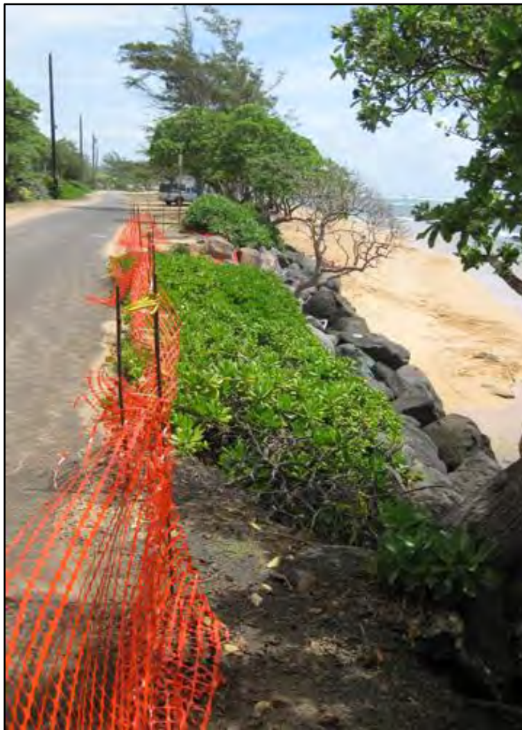
Figure 2-21 View of erosion and fencing looking north from Station 9+10
