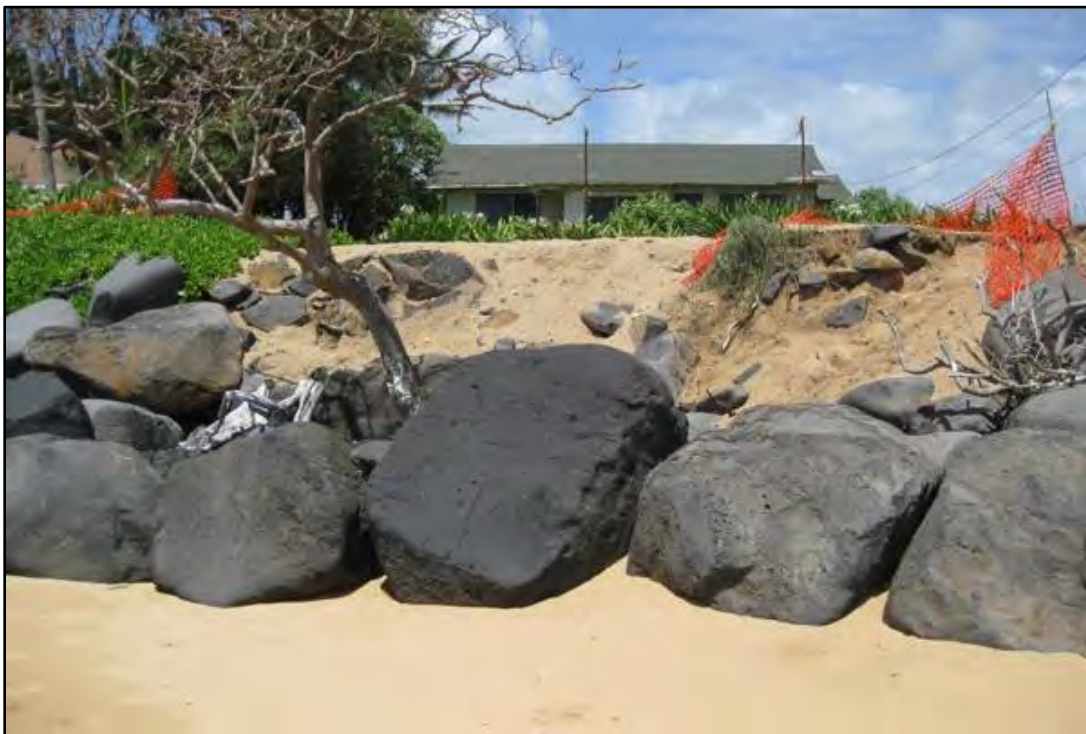
Figure 2-23 View looking west at erosion between Stations 9+70 and 10+00
