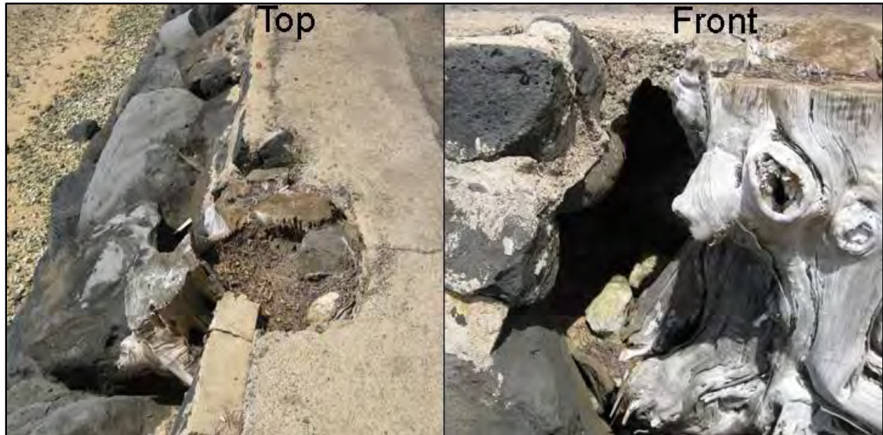
Figure 2-12 Stump and hole in revetment at Station 3+85
