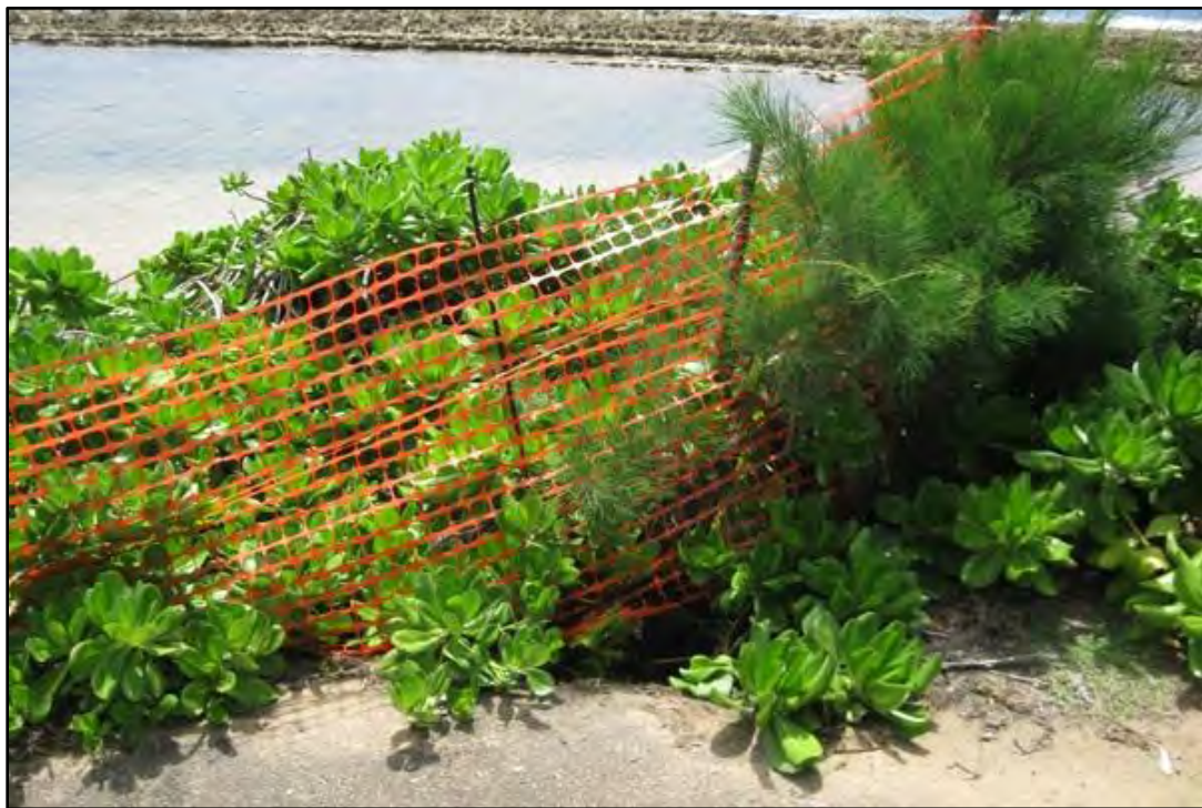
Figure 2-19 View looking east at erosion along roadway at Station 8+20
