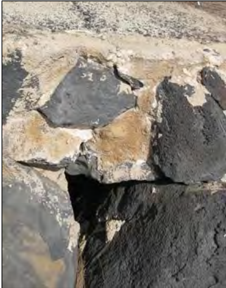
Figure 2-13 Hole at Station 4+50
