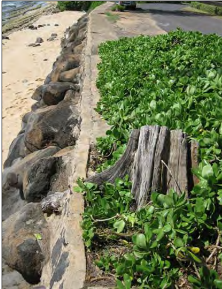
Figure 2-10 Stump in revetment at Station 1+70
