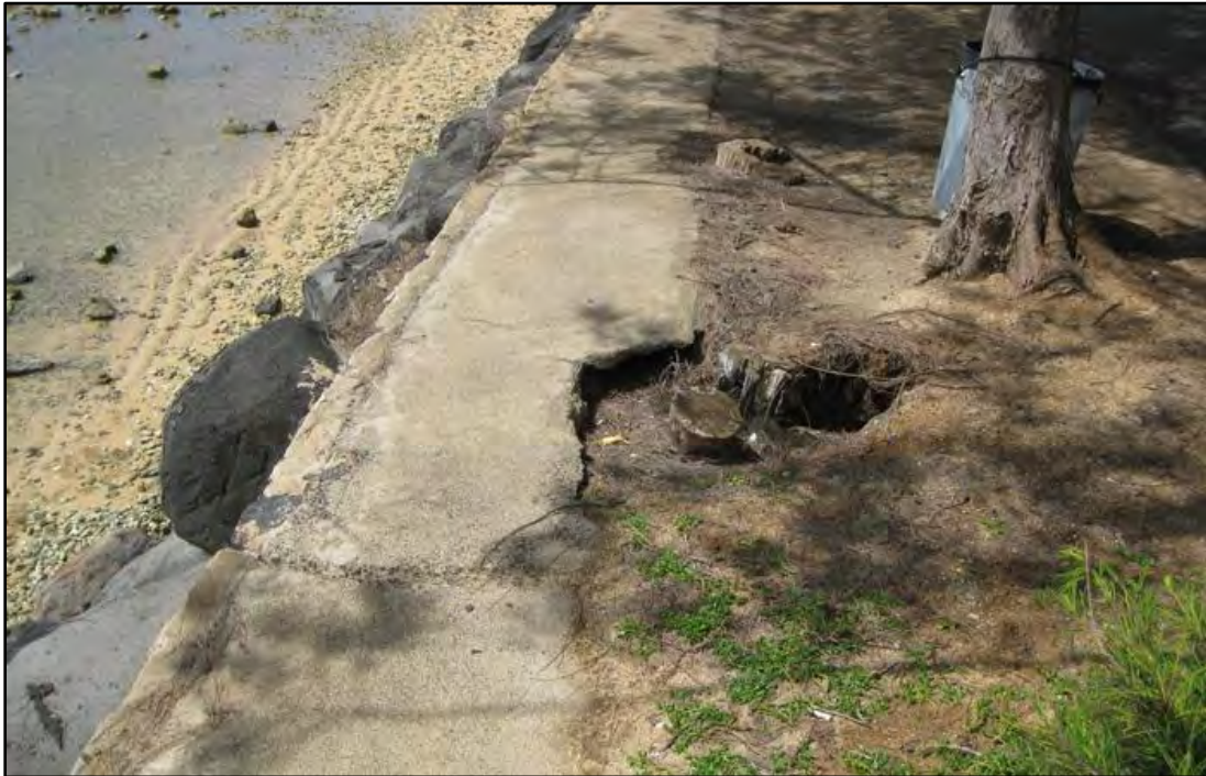
Figure 2-14 Erosion around stumps at Station 4+75
