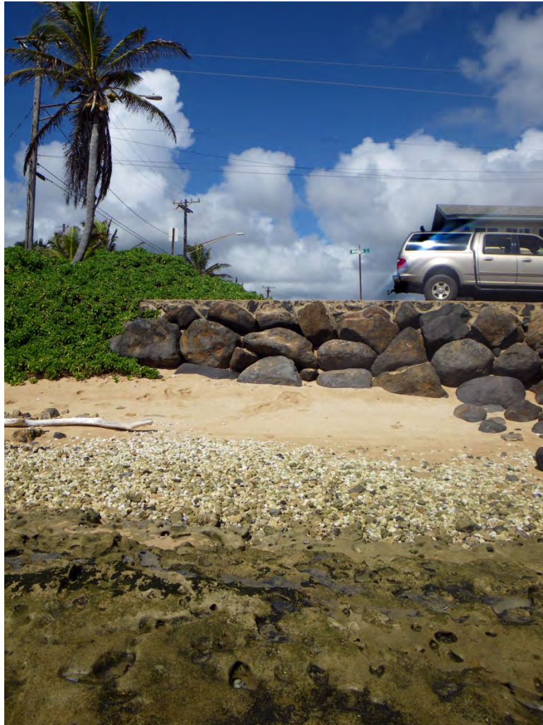
Figure 3. View of south extent of revetment with limestone and narrow beach in foreground.
