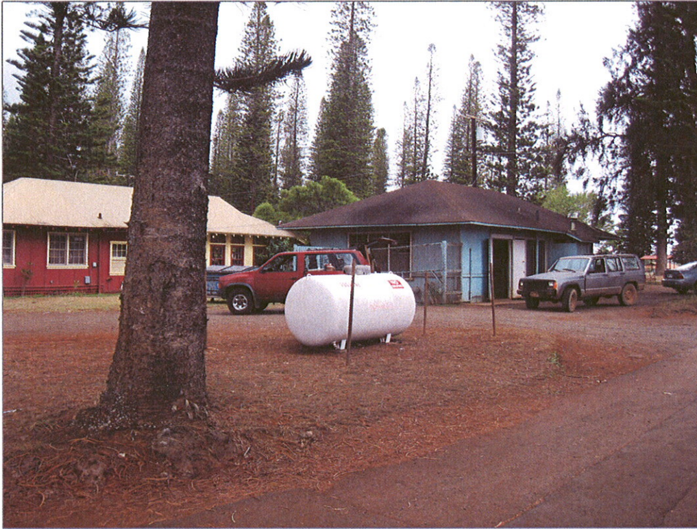
Photo 3: Propane gas tank (499-gallon) behind launderette
