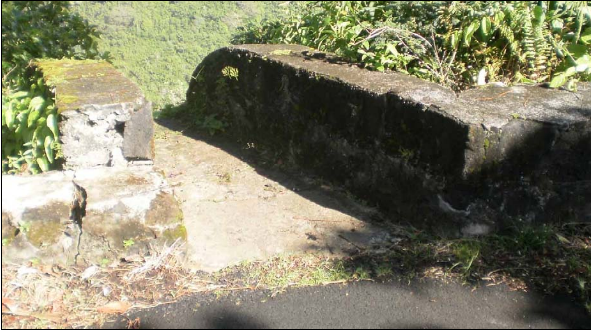
Figure 18. Photograph of the culvert showing the basalt and concrete construction of the sidewalls and the concrete floor, view to northwest
