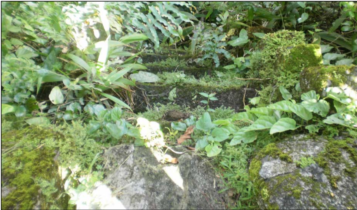
Figure 19. Photograph looking down from the culvert edge showing the concrete cribbing that retains the sediments on this side of the roadway
