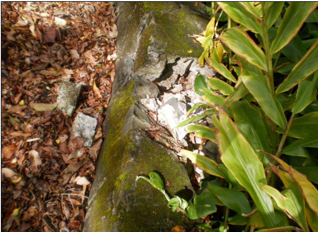
Figure 11. Photograph of a damaged portion of the guard wall showing its internal construction of basalt stones and concrete.
