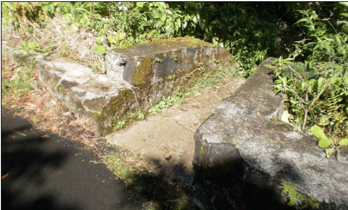
Figure 17. Photograph of the culvert showing the basalt and concrete construction of the sidewalls and the concrete floor, view to southwest.
