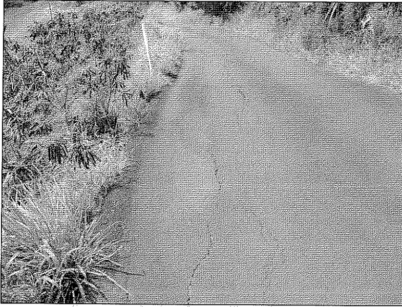
Photo 5: General view of section of damaged roadway, view to southwest.
