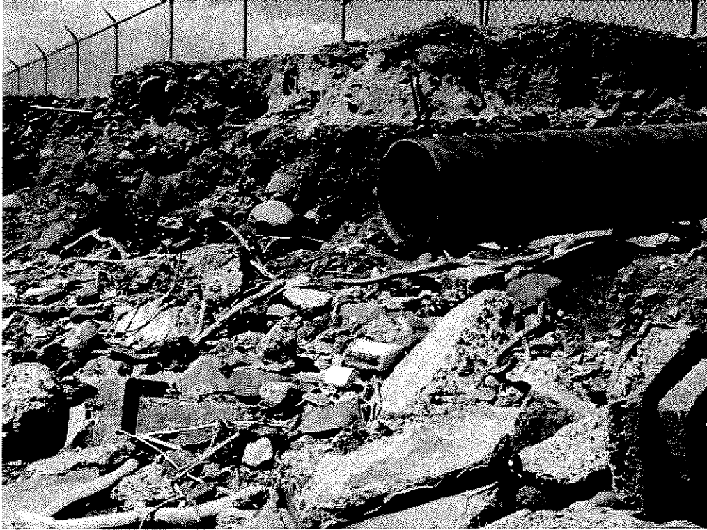
Photo 17. Exposed drainage pipe at the WWPS.
