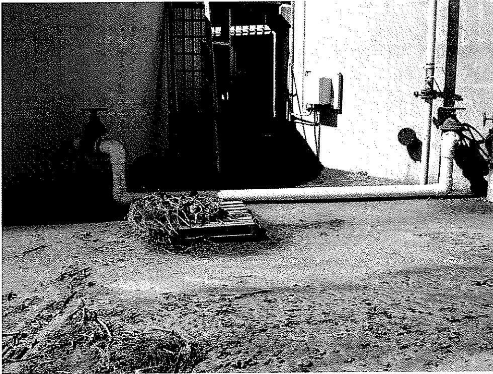
Figure 7. Sand and Debris Near WWRF Sludge Holding Tanks
