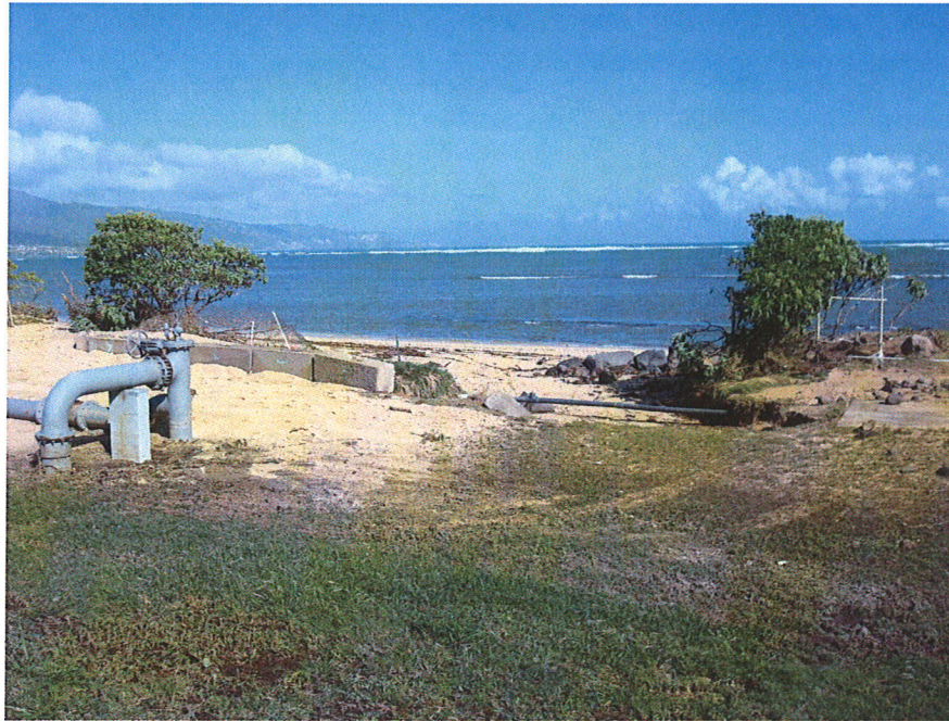
Photo No. 1: Scouring at West End of Revetment (pictured on the right)
