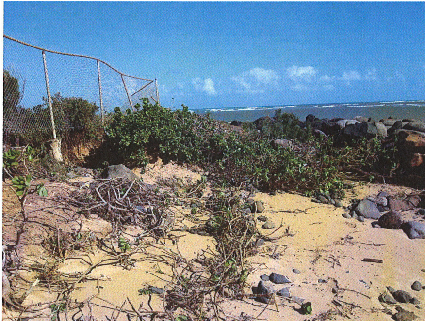
Photo No. 2: Erosion from Behind the East Flank, Which Undermined the Chain Link Fence Footings
