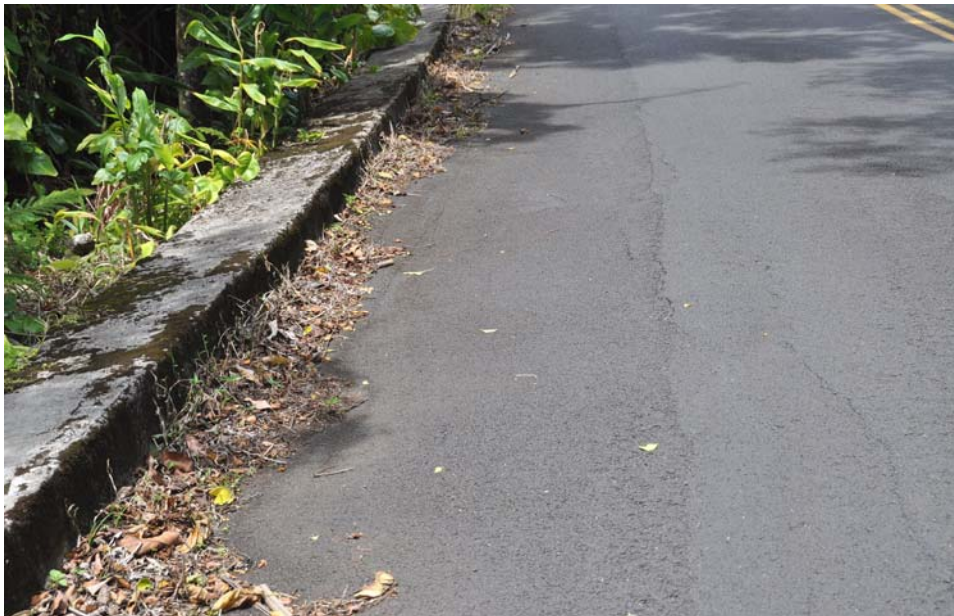
Photo 3. CRM wall slanting toward Makiki Valley, pavement cracks in roadway
