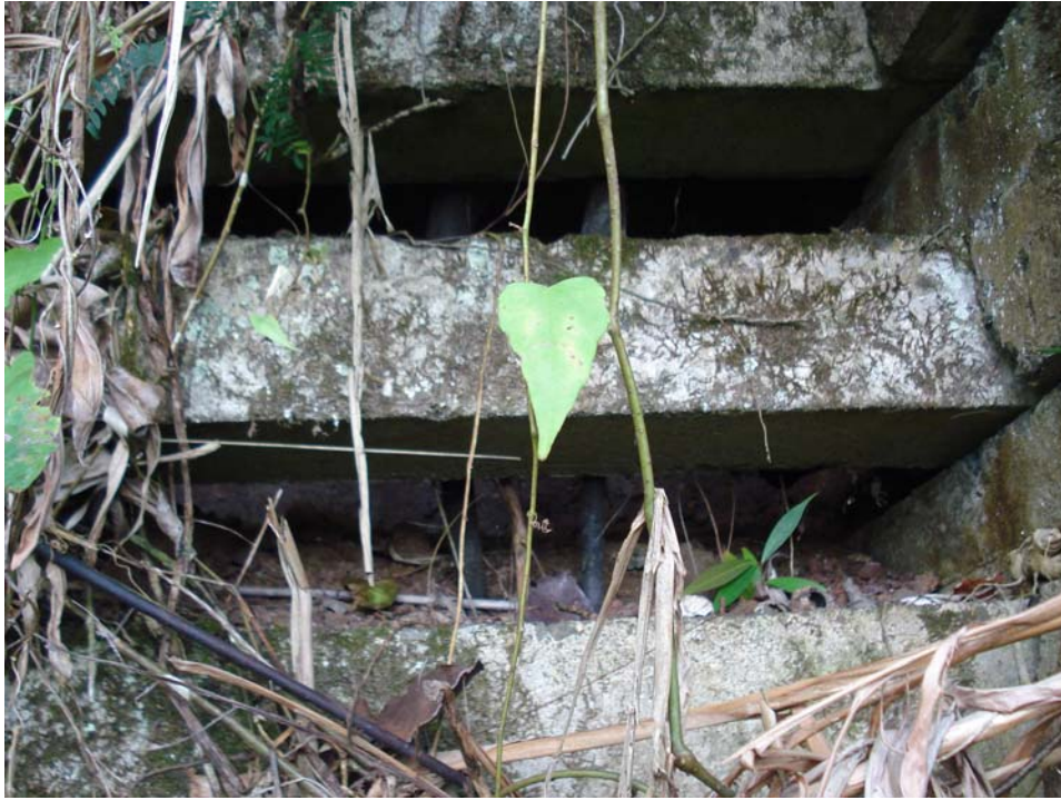
Photo 6. Close-up of crib wall shows erosion of fill material
