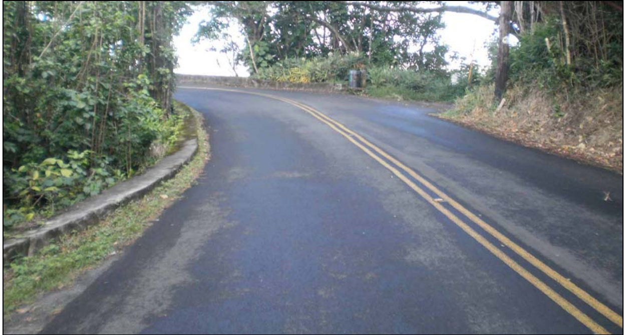
Figure 12. Photograph showing the low curb on the southeastern (Makiki Valley) side of Tantalus Drive at the north end of the project area, view to west
