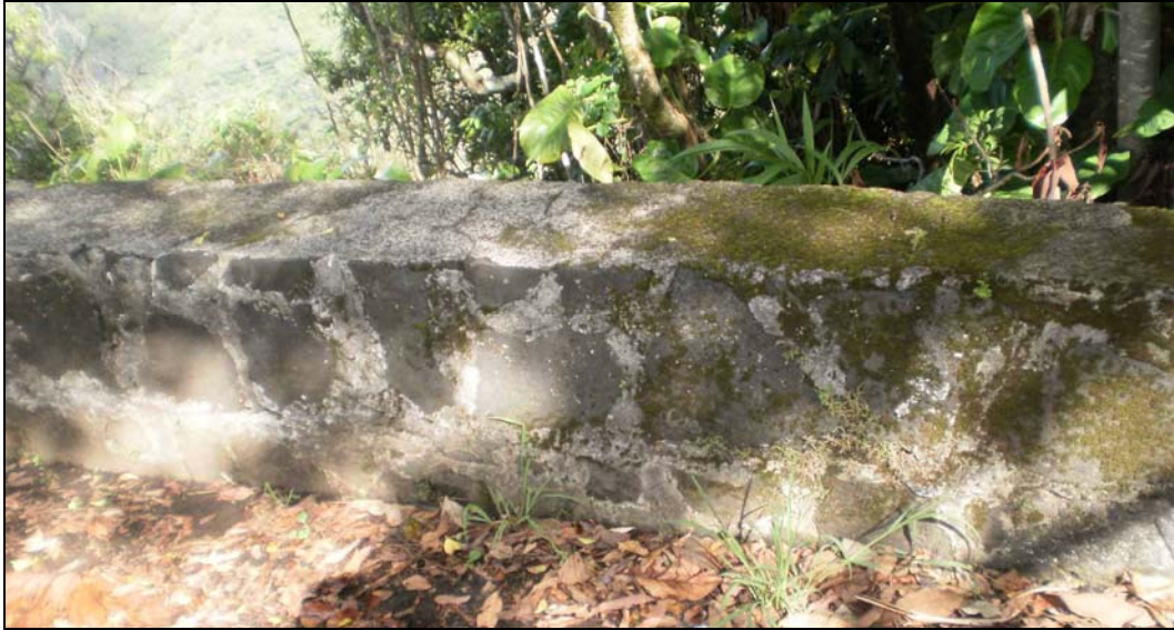
Figure 10. Photograph of the guard wall showing its construction of basalt and concrete, with a smooth concrete top, view to west.
