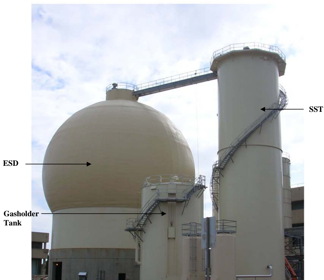
Figure 2-4, Photo of Existing ESD/SST and Gasholder Tank, Sand Island WWTP (Source: CB&I)
