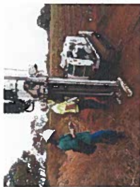
ETC personnel beginning the subsurface sample collection with the track drill rig
