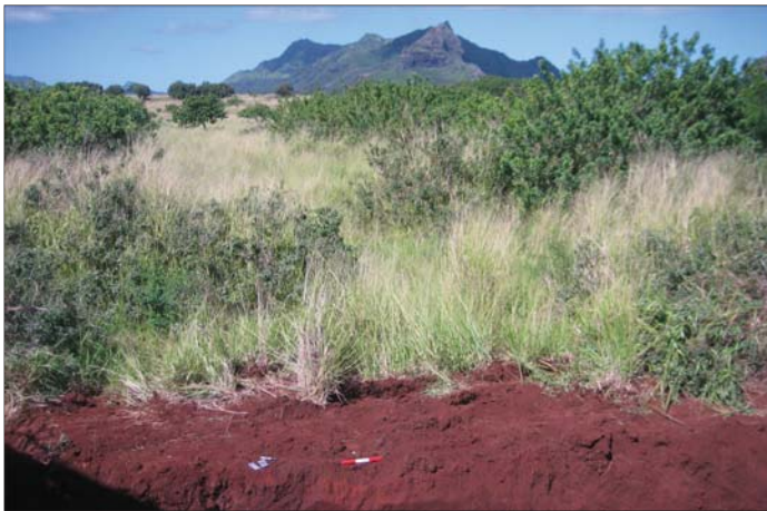
Figure 18: Photograph of the backhoe excavation of Trench 10, looking northwest. The northeast wall of Trench 10 is in the foreground, below the bar scale. Kalalea Mountain is in the background. The scale is in ten centimeter increments.
