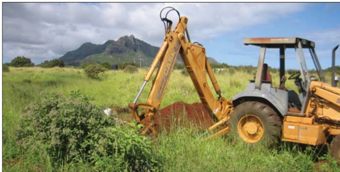
Figure 8: Photograph of the backhoe excavation of Trench 1, looking northwest. Kalalea Mountain is in the background.
