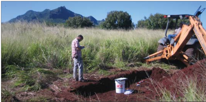
Figure 11: Photograph of the backhoe excavation of Trench 3, looking northwest. Kalalea Mountain is in the background.
