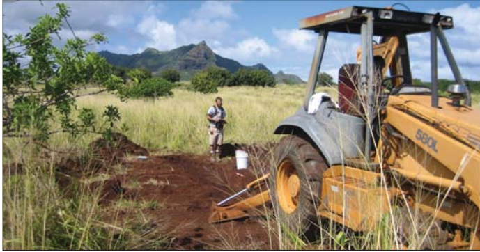
Figure 13: Photograph of the backhoe excavation of Trench 5, looking northwest. Kalalea Mountain is in the background.
