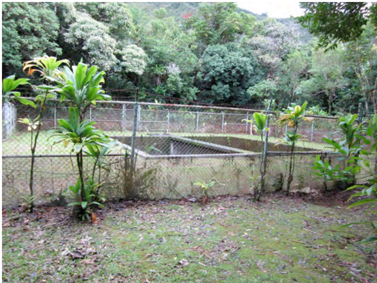
Photo 11: Sand filters are located within secure enclosure.
