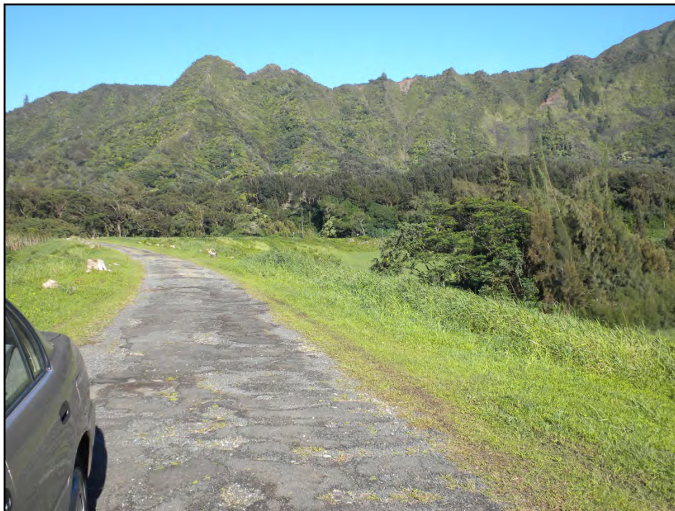
Figure 50. Portion of reservoir access road, view to the northwest (towards the Pali Highway)
