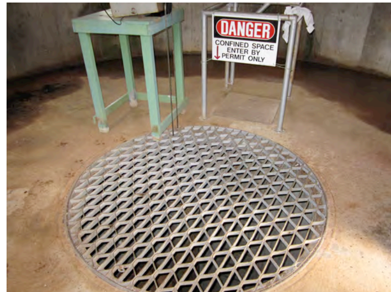
Photo 8: Access to sluice gates below control room is via confined space entry.
