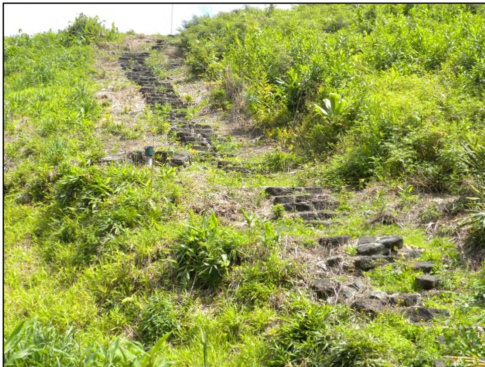
Figure 48. Paved trail leading up the embankment dam from the outlet receiving area
