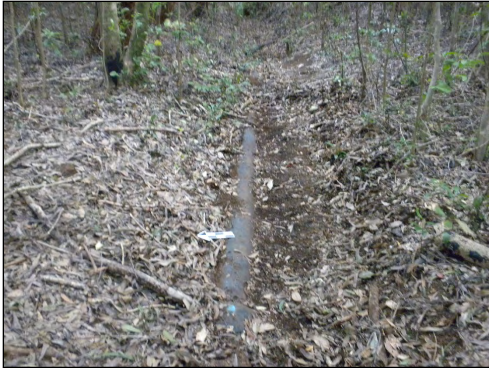
Figure 38. Partially-buried metal pipe within level area of ditch
