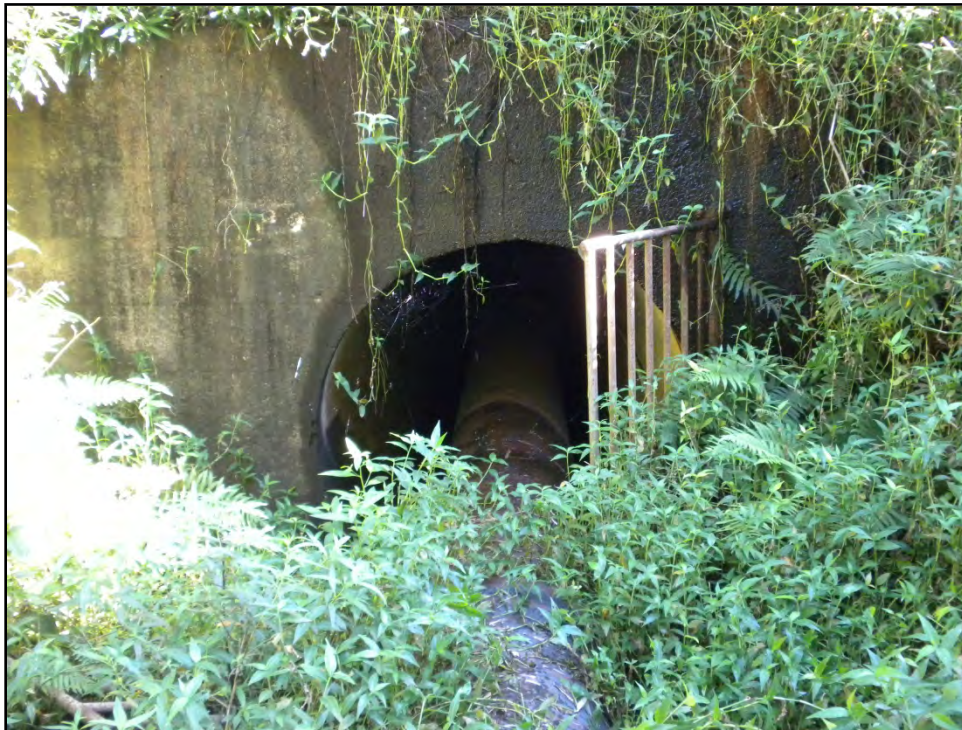
Figure 46. Outlet receiving area with 24-inch pipe coming out of the downstream slope of the embankment dam
