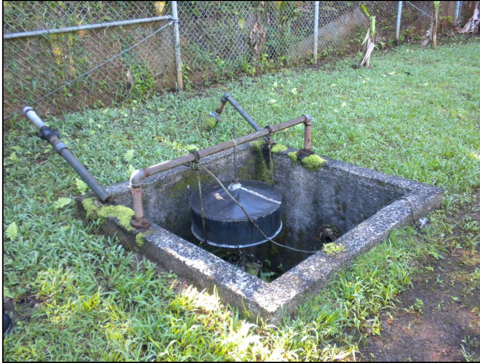
Figure 53. Part of water filtering system
