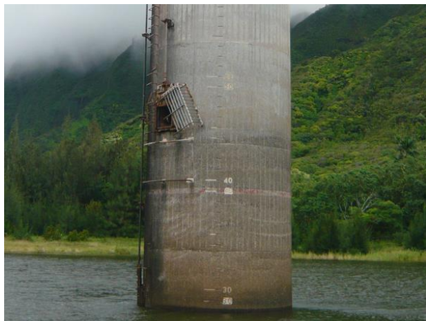
Figure 2-9: Top Gate and Trash Rack.
