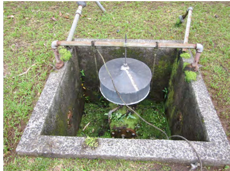
Photo 12: Float valve for sand filters at Nuuanu Reservoir #4.
