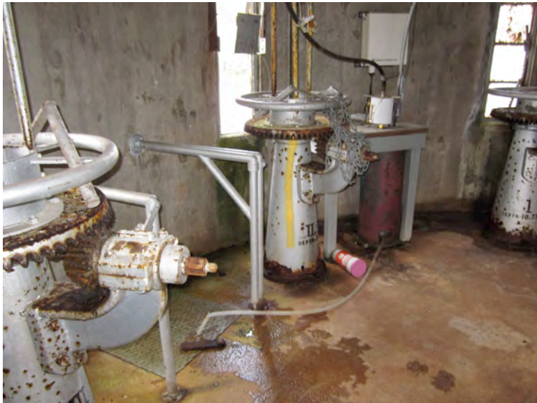
Photo 5: Inlet control valves inside control room of intake tower at Nuuanu Reservoir #4.
