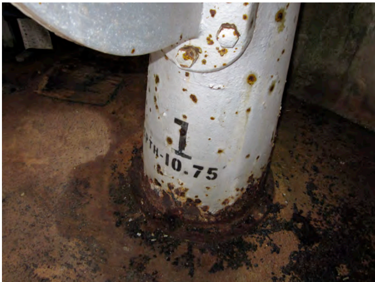
Photo 7: Painted surfaces on valves is rusting and in poor condition.
