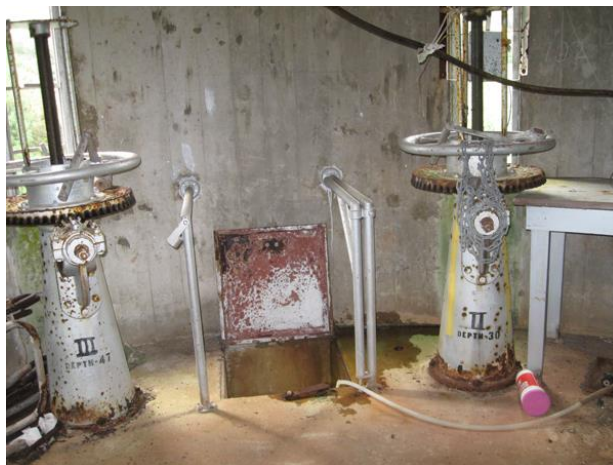
Figure 2-10: Intake Tower Gate Controls.
