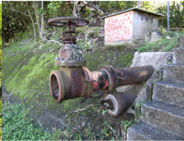
Figure 3-12: Water Valves (no longer used)
