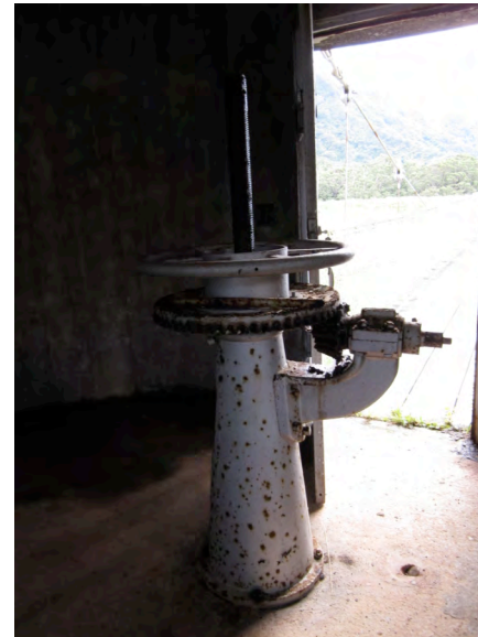
Photo 6: Outlet control valve.
