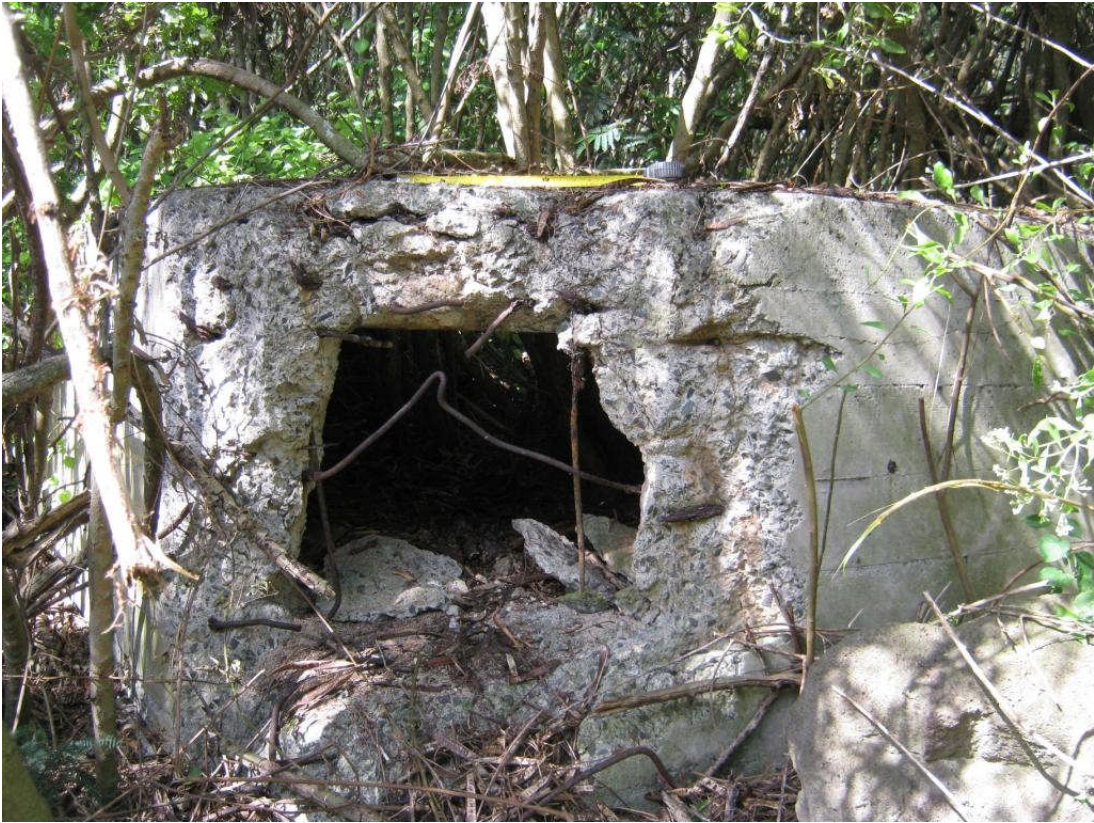
Figure 83. Site 7287 displaced concrete structure remnant, view to northeast
