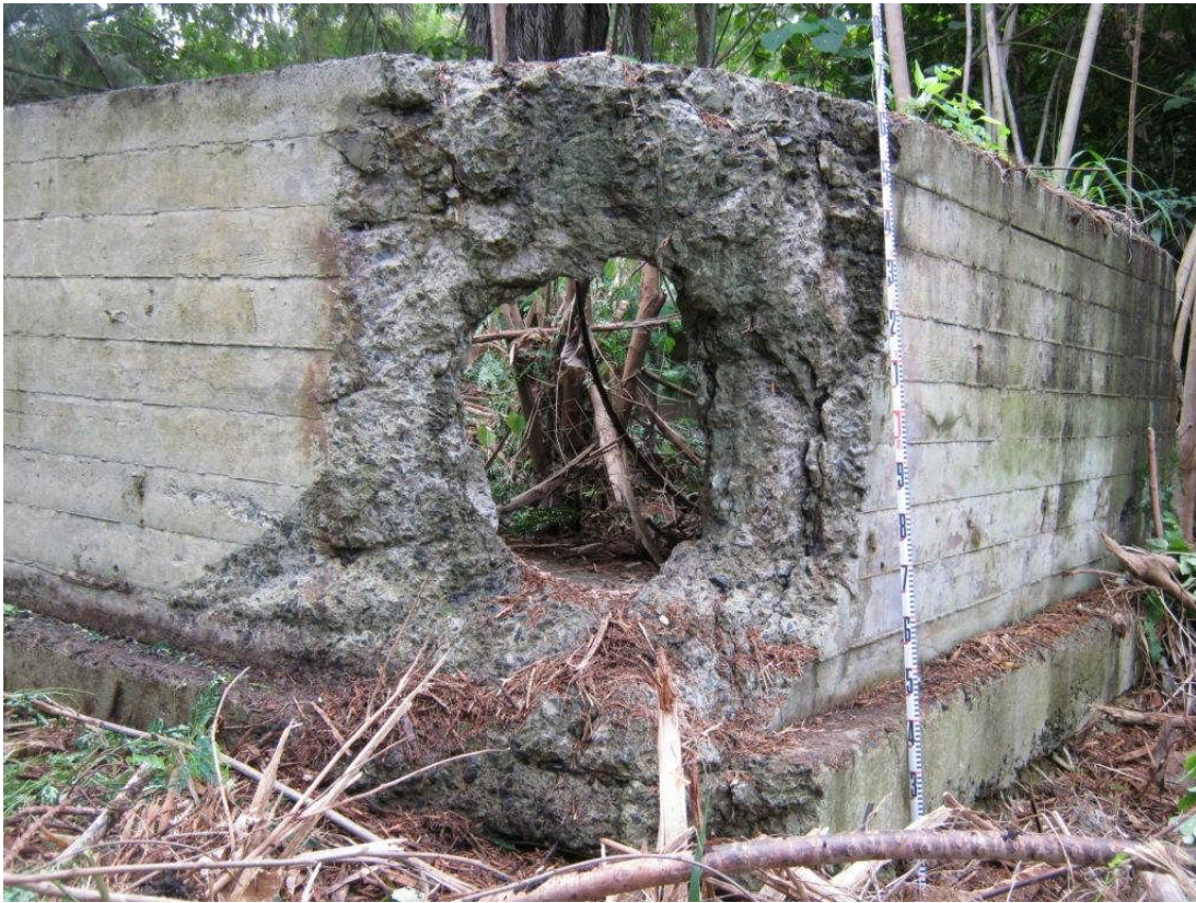
Figure 50. Site 7278 blown out corner of concrete structure, view to southwest
