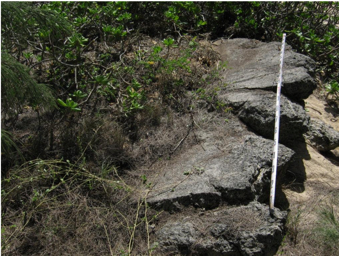
Figure 15. Site 7262 disturbed concrete slab, view to west
