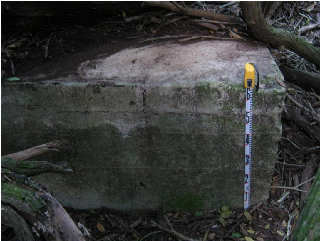
Figure 74. Corner of Site 7284, Feature C showing form board marks, view to northeast
