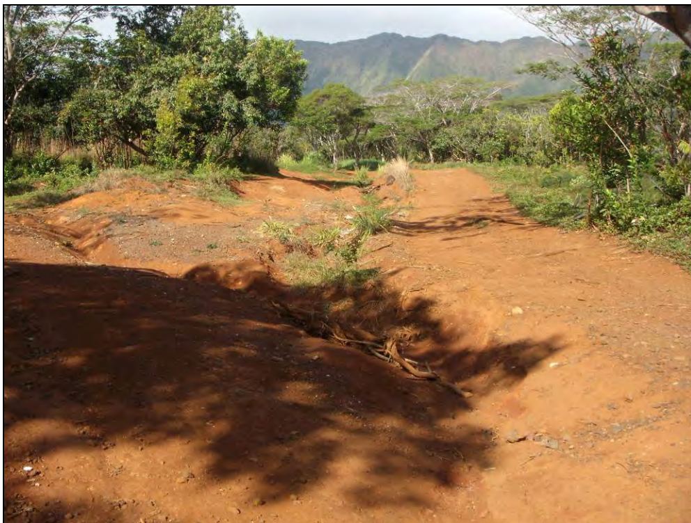
Figure 13. Erosion impacted roadway in the NPA, view to the west
