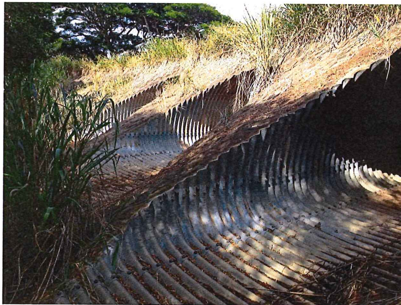
Figure 9. Culverts provide passage for freshets under Makani Road, though the gulch up and down from the road is indistinct from the surrounding landscape.
