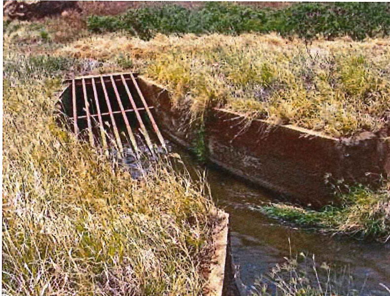
Figure 7. Haiku Ditch entering a siphon under Kailua Stream, approximately 2167 m (7110 ft) upstream from Hāna Highway (April 2011).
