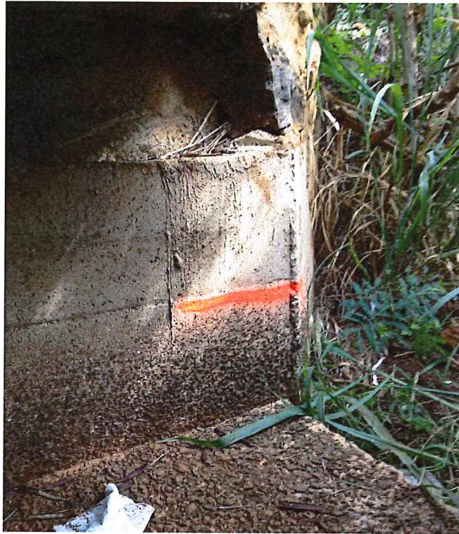
Figure 12. Eroded concrete below the OWHM (orange line) within the existing culvert under Hāna Highway (November 2013).
