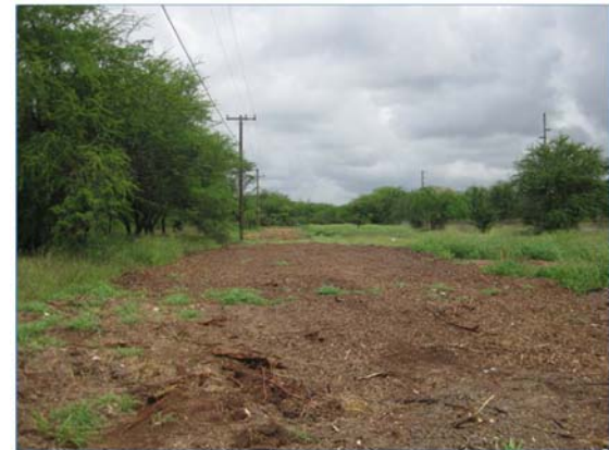
Fig. 10. The Corridor bordering the Honouliuli WWTP was recently cleared by a forestry mower and is covered with kiawe chips.
