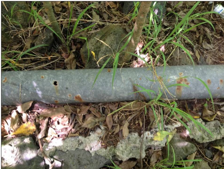
Figure 5. Hole in the 6-inch Pipe
