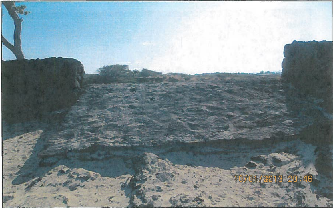
PHOTO 3: Existing stone/ concrete ramp to be demolished and new stairway to be constructed in its place, view to the E.
