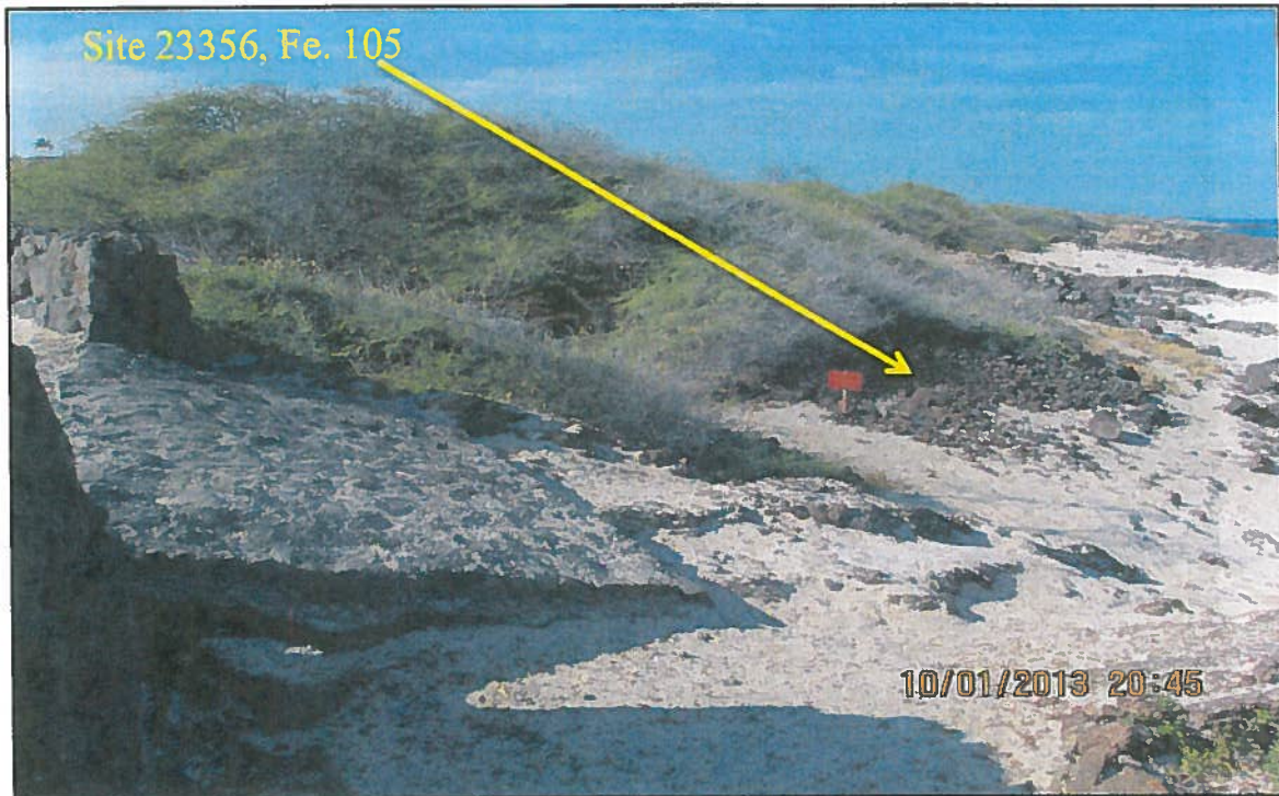
PHOTO 4: Existing stone/ concrete ramp to be demolished, and new stairway to be constructed in its place, view to the S. NOTE: SIHP Site 23356, Feature 105 in the background.
