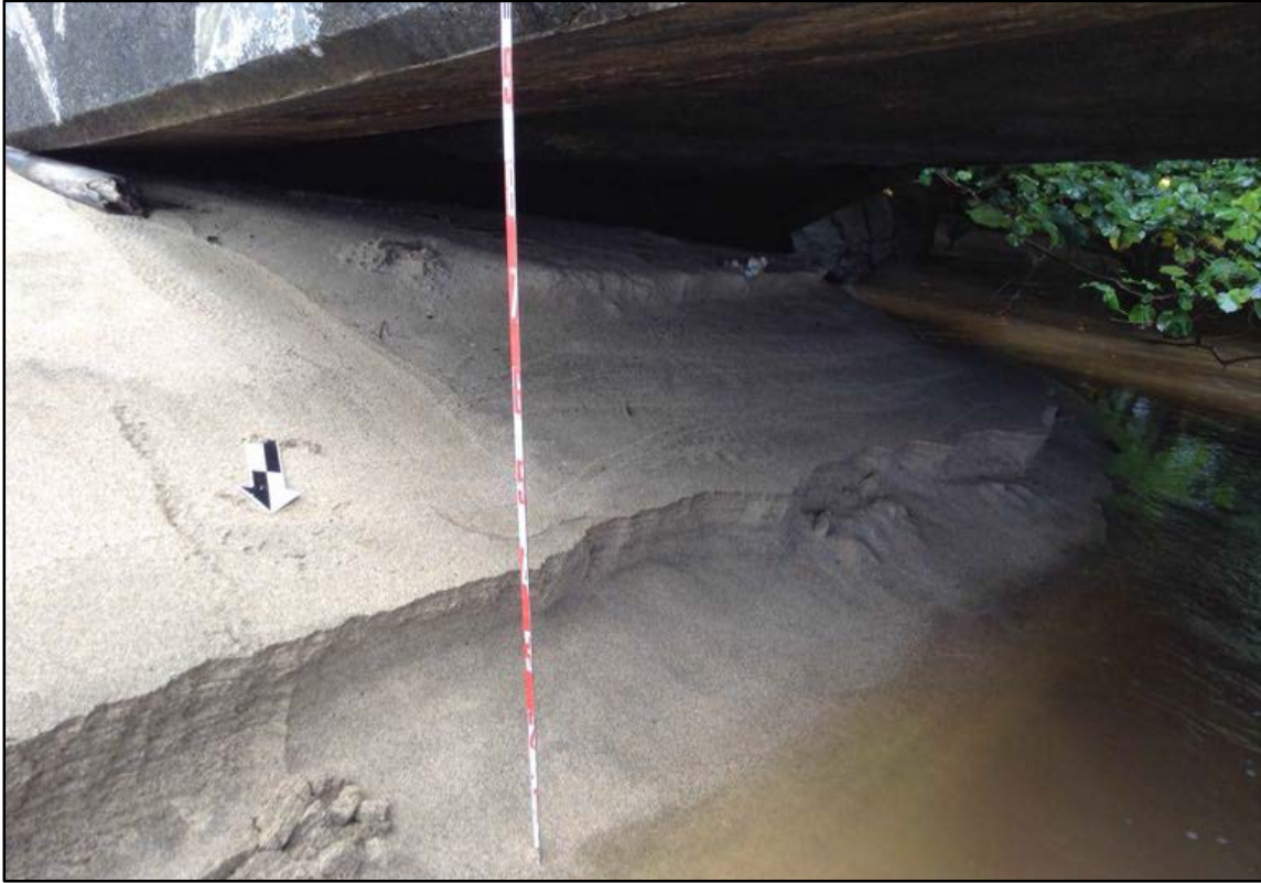
Figure 64. SIHP # 50-30-03-2298, the Waikoko Stream Bridge, underneath profile view to south of the 1912 portion of the bridge undermined by the 1946 tsunami
