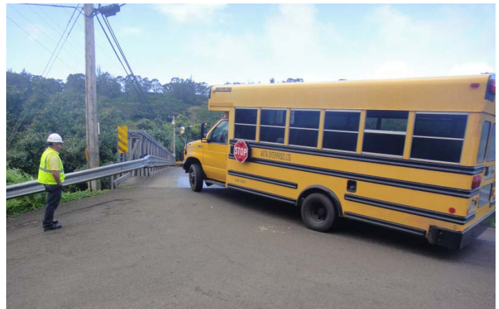
Resiliency and maintenance of structure from regular use is a consideration, especially due to the tight navigation
