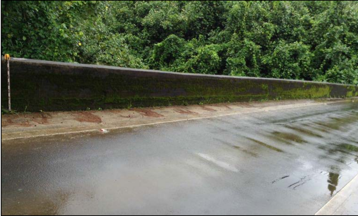
Figure 53. SIHP # 50-30-03-2297, the Waipā Stream Bridge, portion of the 1925 extension, profile view to west
