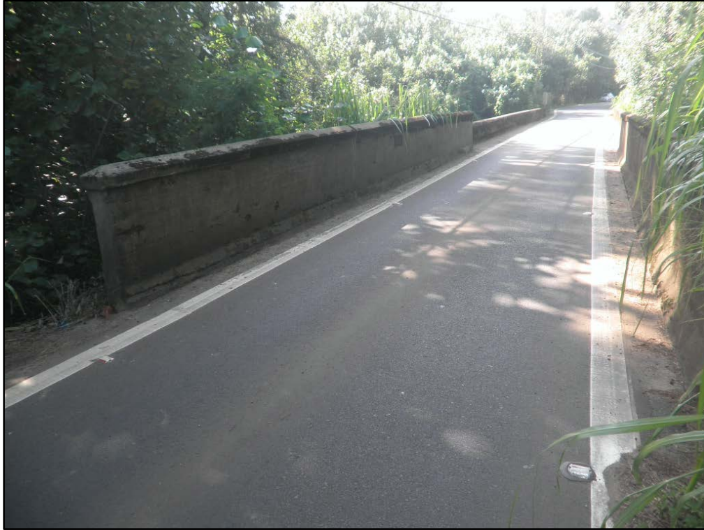
Figure 51. SIHP # 50-30-03-2297, the Waipā Stream Bridge, general view to northwest; note the 1912 bridge portion in the foreground
