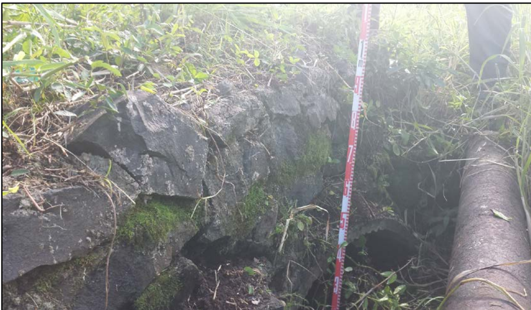
Figure 72. Portion of SIHP # 50-30-02-2299, road culvert and revetment northeast of Wainiha Bridge 2, outflow end (at lower right) on the west side of the road, view to south
