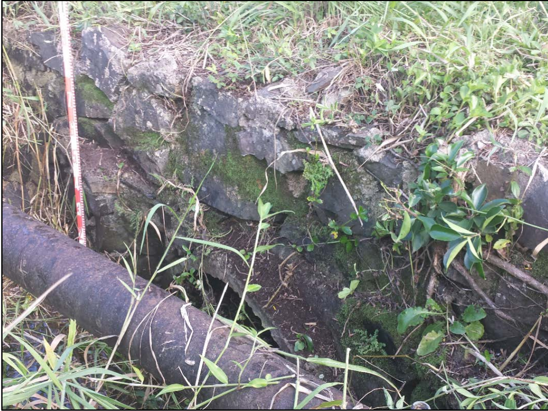
Figure 71. SIHP # 50-30-02-2299, road culvert and revetment northeast of Wainiha Bridge 2, outflow end on the west side of Kūhiō Highway, view to northeast
