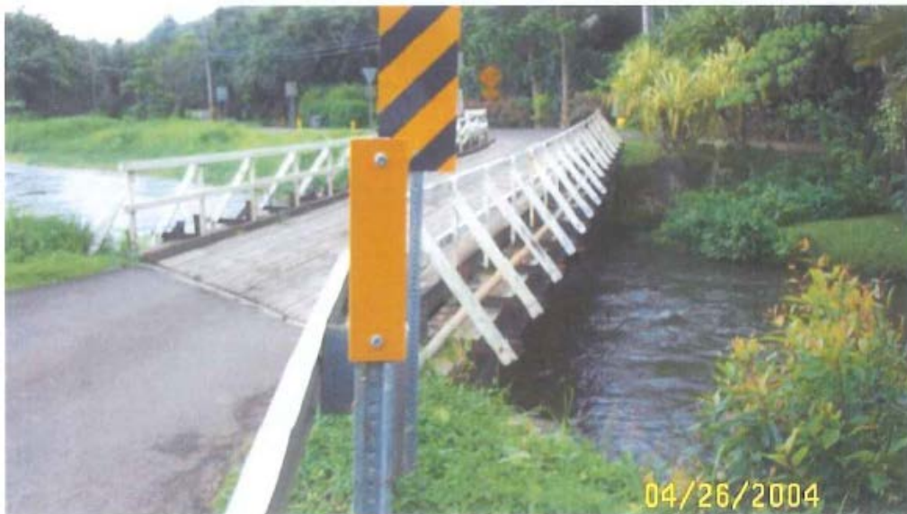
Photo 6: View of historical Bridge 2 from western approach, mauka side, looking east toward Lihue (before replacement with ACROW bridge in 2004) (HDOT 2012)
