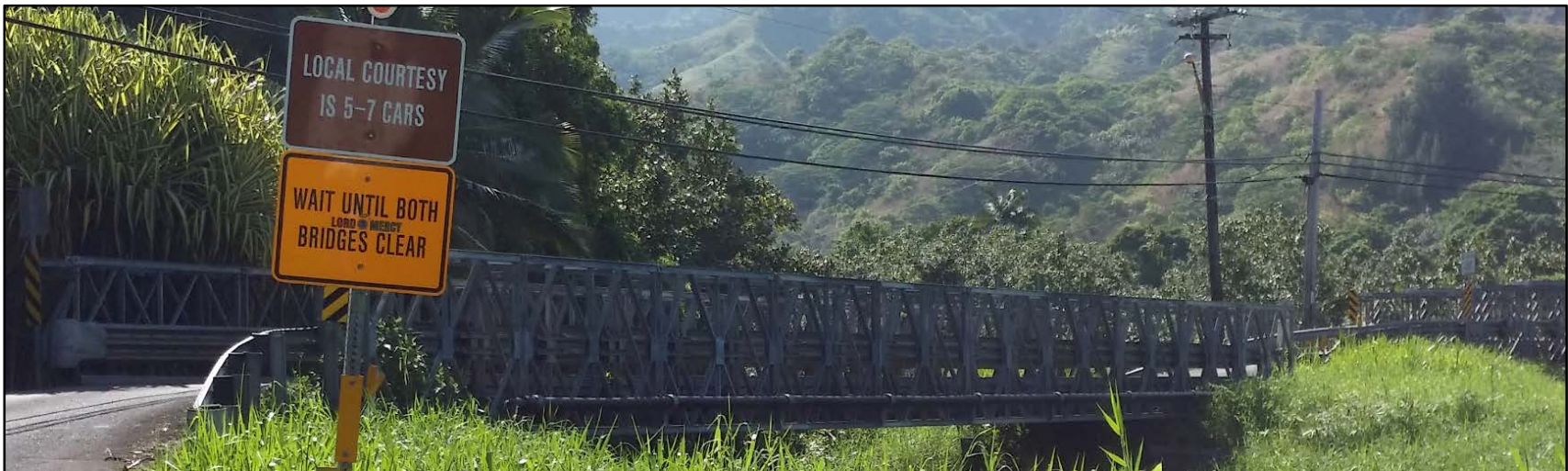
Figure 40. Portion of the Kūhiō Highway, view to south of Wainiha Bridge 2; note sign indicating the local custom of taking turns to cross the bridge, allowing 5-7 cars across at a time
