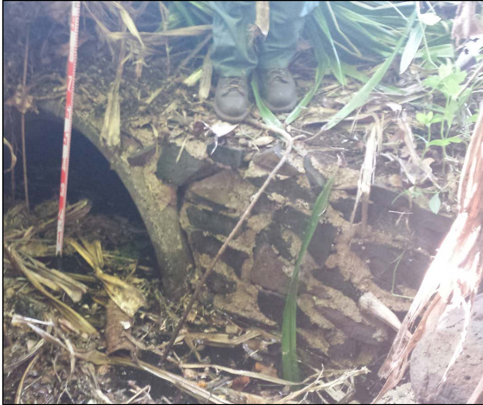
Figure 73. SIHP # 50-30-02-2299, intake portion of the road culvert and buttressing northeast of Wainiha Bridge 2, on the east side of Kūhiō Highway, view to southwest
