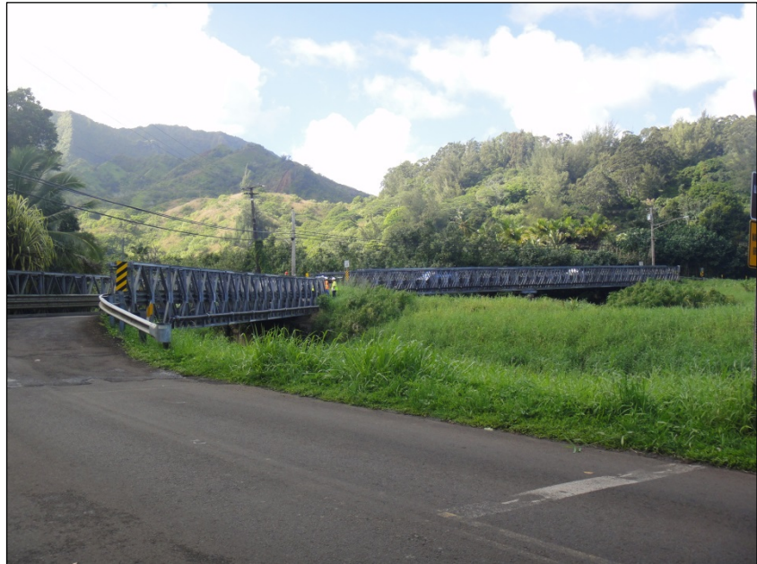
Photo of existing Bridges 2 and 3 and how they operate as one bridge
