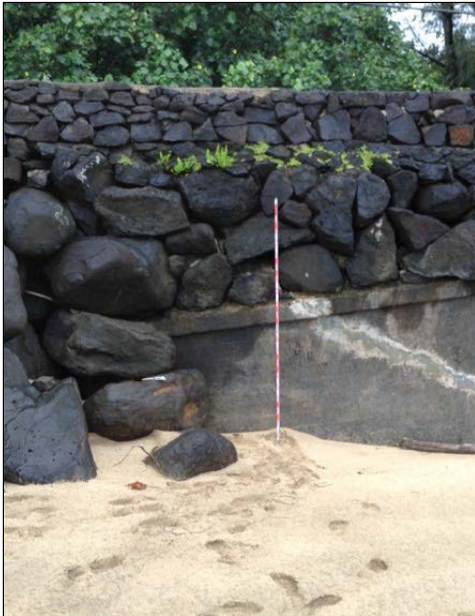
Figure 66. SIHP # 50-30-03-2298, the Waikoko Stream Bridge, profile view to southwest; note the 1912 portion of the bridge undermined by the 1946 tsunami, with portions of the basalt base course and overlying basalt boulder and mortar repair
