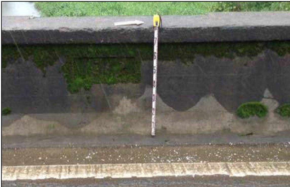
Figure 48. SIHP # 50-30-03-2296, the Wai'ole Stream Bridge, profile view to west, showing concrete stamped "1912"
