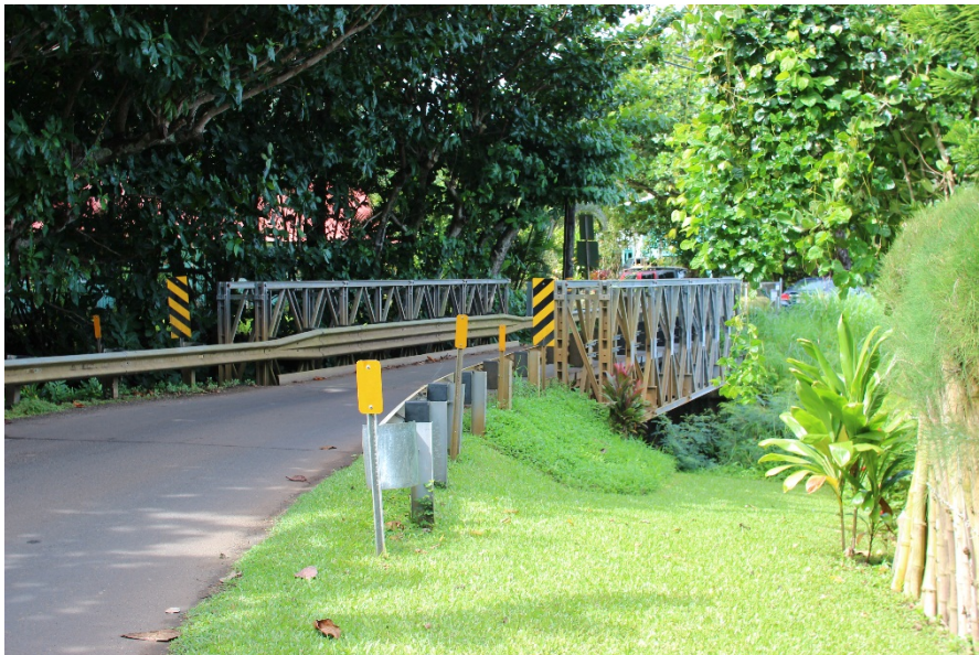
Photo 1: View of existing Wainiha Bridge 1 from eastern approach, makai side, looking west toward Hā'ena (from Kūhiō Highway).
