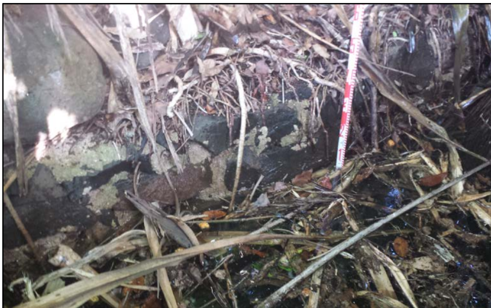
Figure 74. SIHP # 50-30-02-2299, road culvert northeast of Wainiha Bridge 2, portion of the intake revetment on the east side of Kūhiō Highway, view to southeast
