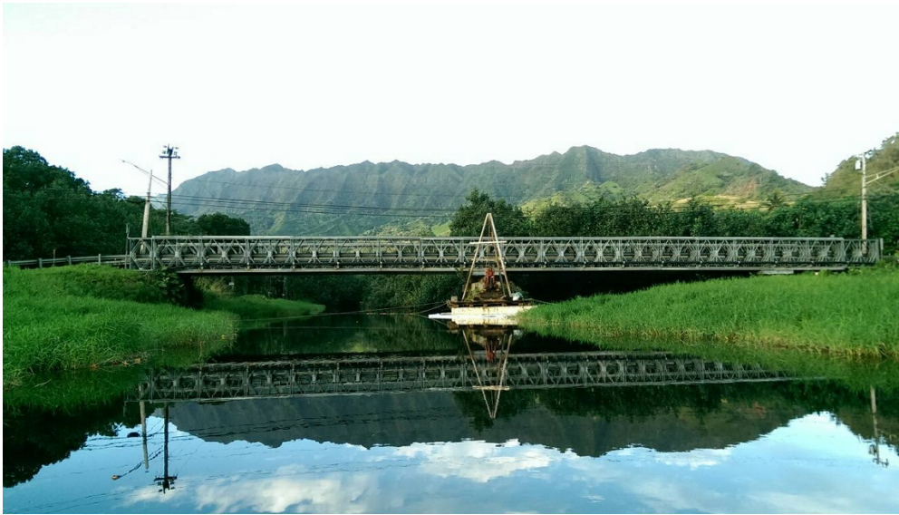
Photo 4: View of existing Wainiha Bridge 3 from Wainiha River, makai side, looking southwest, upstream (a drill rig is in front of the bridge).
