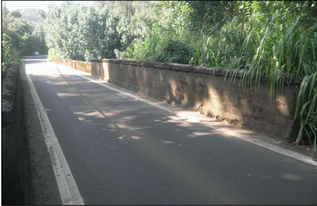
Figure 55. SIHP # 50-30-03-2297, the Waipā Stream Bridge, view to north; note the 1912-built bridge portion in the foreground
