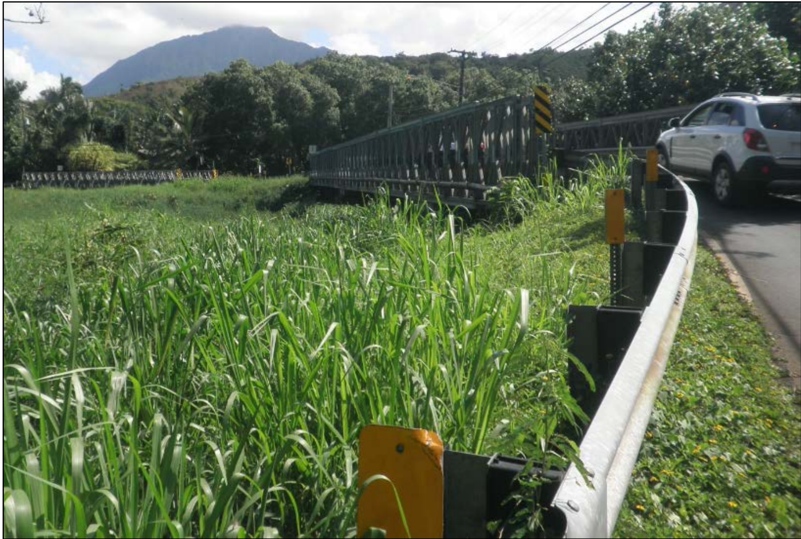
Figure 43. A portion of the Kūhiō Highway, Wainiha Bridges 3 and 2 respectively, non-contributing structures within the historic bridges district, general view to southeast with Pu‘uuhia in the background
