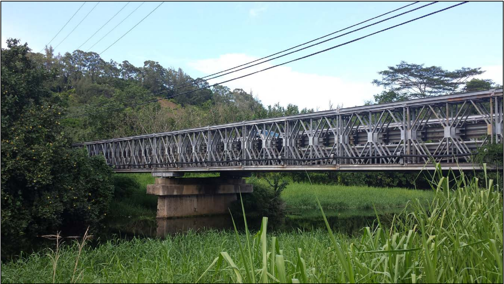
Figure 42. A portion of the Kūhiō Highway at the Wainiha Bridge 3, a non-contributing structure within the historic bridges district, general view to north
