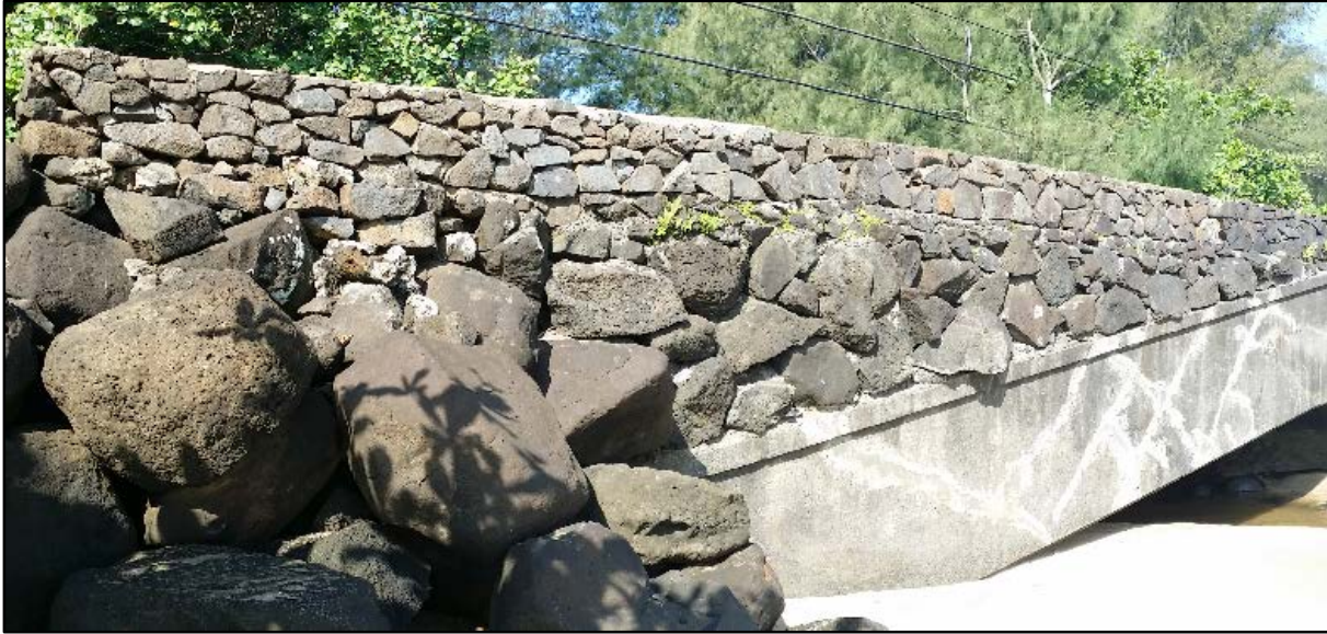
Figure 60. SIHP # 50-30-03-2298, the Waikoko Stream Bridge, general view to west of the bridge's makai face; note approximately eight courses of basalt boulders mortared on top of the concrete portion of the bridge damaged in the 1946 tsunami
