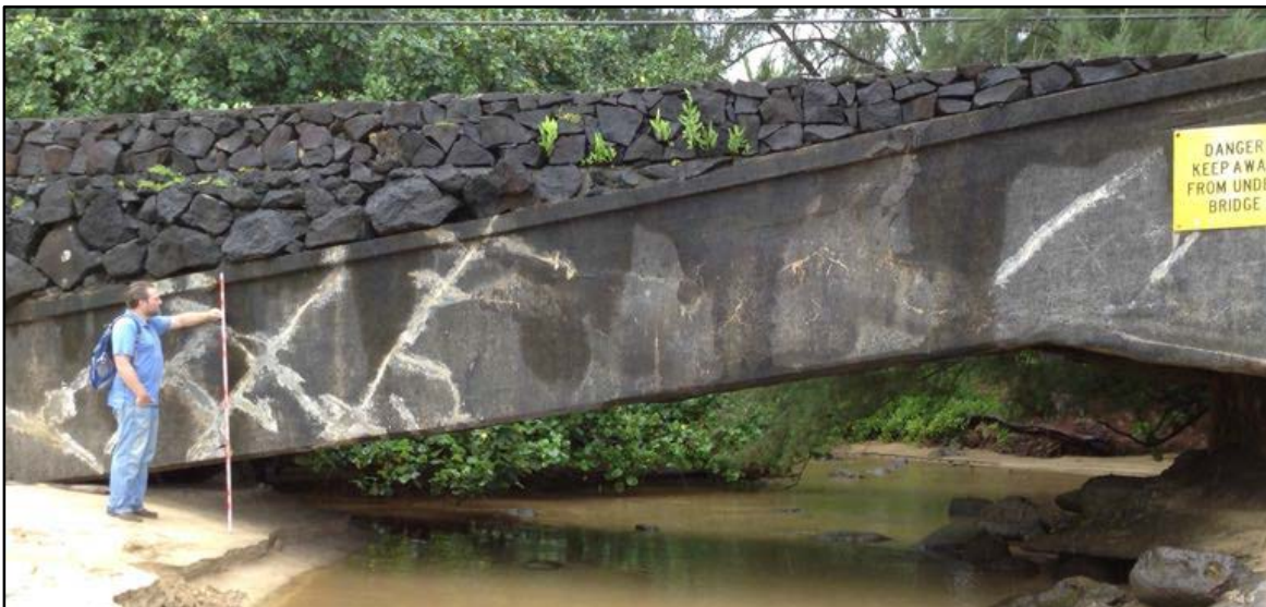
Figure 65. SIHP # 50-30-03-2298, the Waikoko Stream Bridge, profile view to southwest; note the 1912 portion of the bridge undermined by the 1946 tsunami, with portions of the overlying basalt boulder and mortar repair
