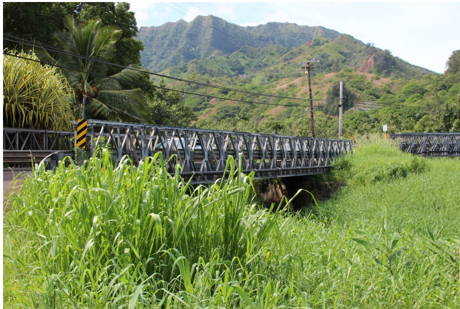
Photo 2: View of existing Wainiha Bridge 2 from the eastern approach, makai side, looking west toward Hā'ena (eastern end of Wainiha Bridge 2 is visible in the background on the right side of the photo) (from Kūhiō Highway).
