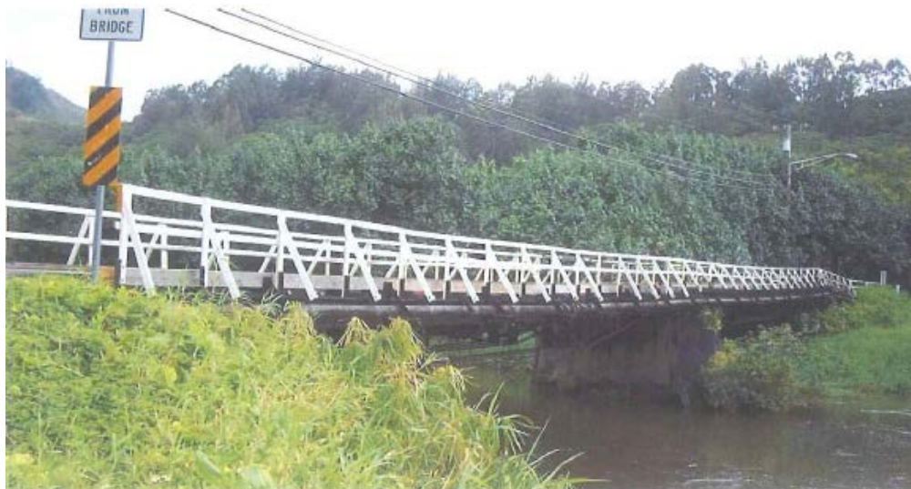
Photo 7: View of historical Bridge 3 from western approach, mauka side, looking east toward Lihue (before replacement with ACROW bridge in 2007) (HDOT 2012)
