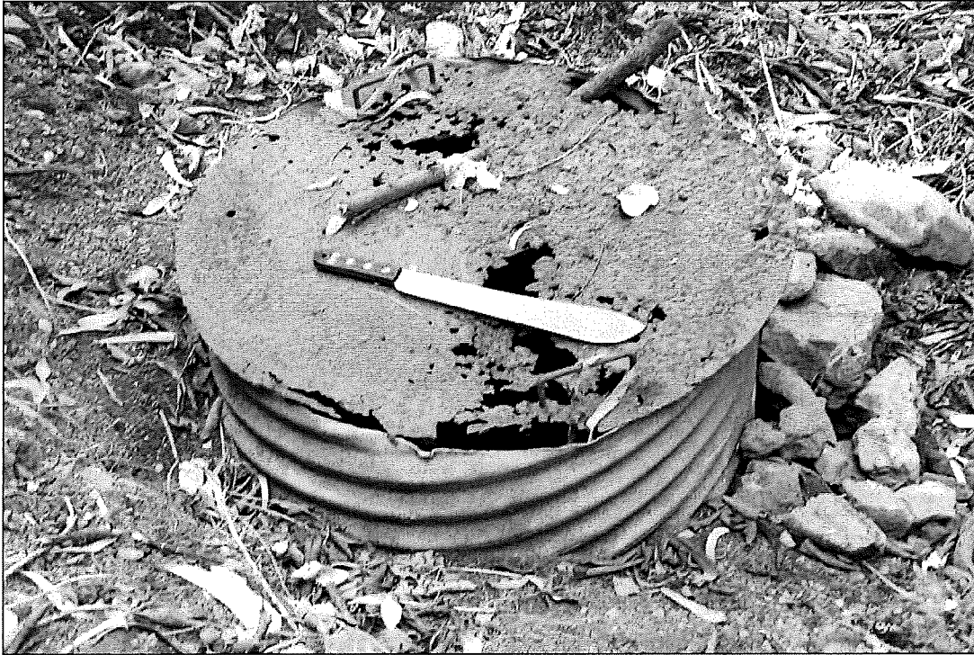
Figure 12. Corrugated pipe containing a water valve.
