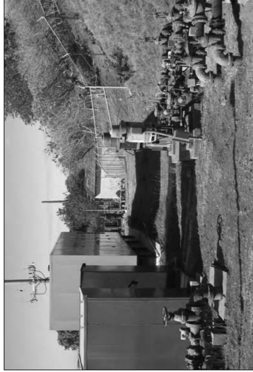
Figure 6. Project Area 1, wells, booster pumps and generators (view south).
