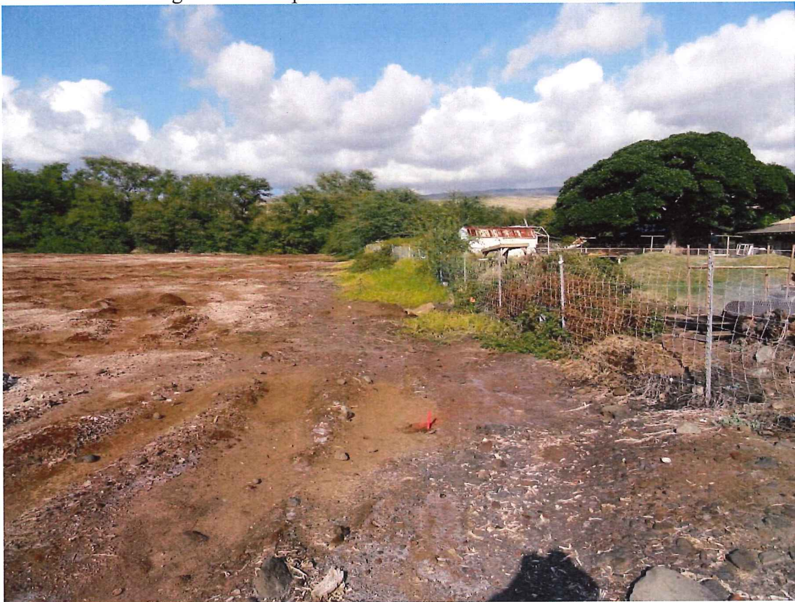
Figure 16. View north along the project boundary. The proposed wetland boundary is indicated by red stakes which are located near the toe of the slope below the elevated DHHL houselots.
