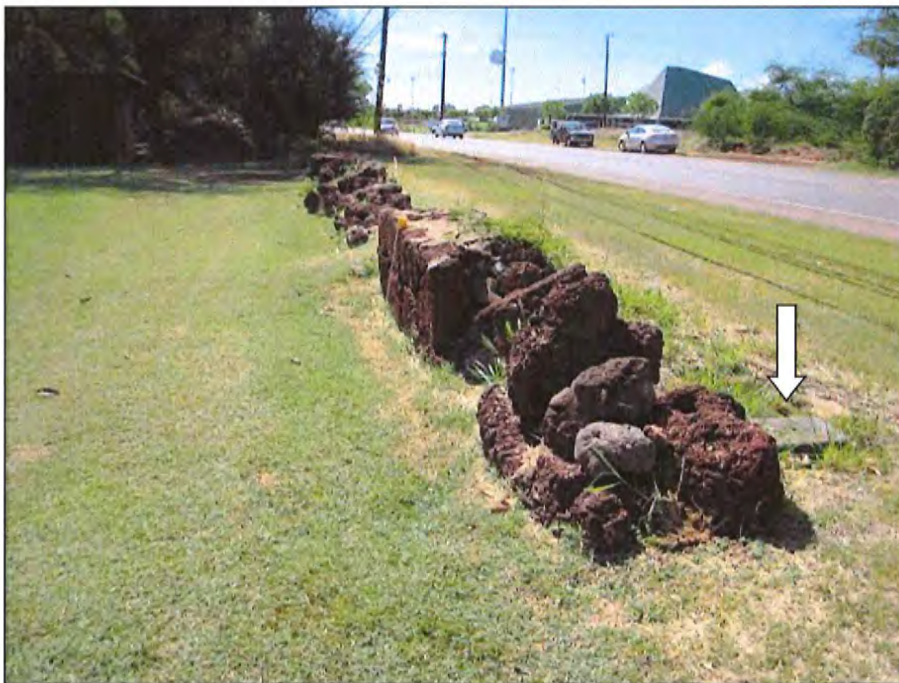
Figure 14. Degraded section of wall in project area, facing west. Arrow indicates location of valve box.
