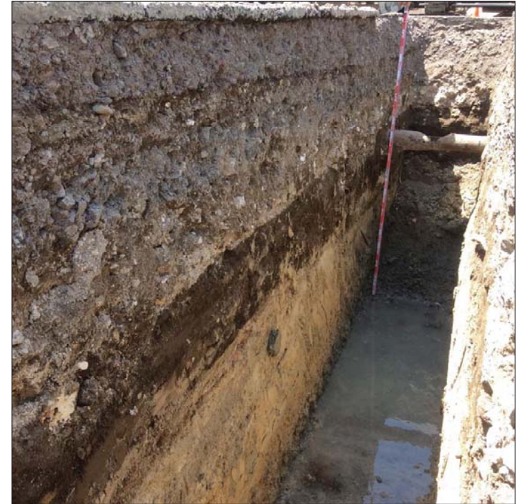
Figure 42. Photograph of T-3 southwest wall showing sewer pipe at 80 cmbs and wetland sediments (Stratum IV) visible in northwest end of trench
