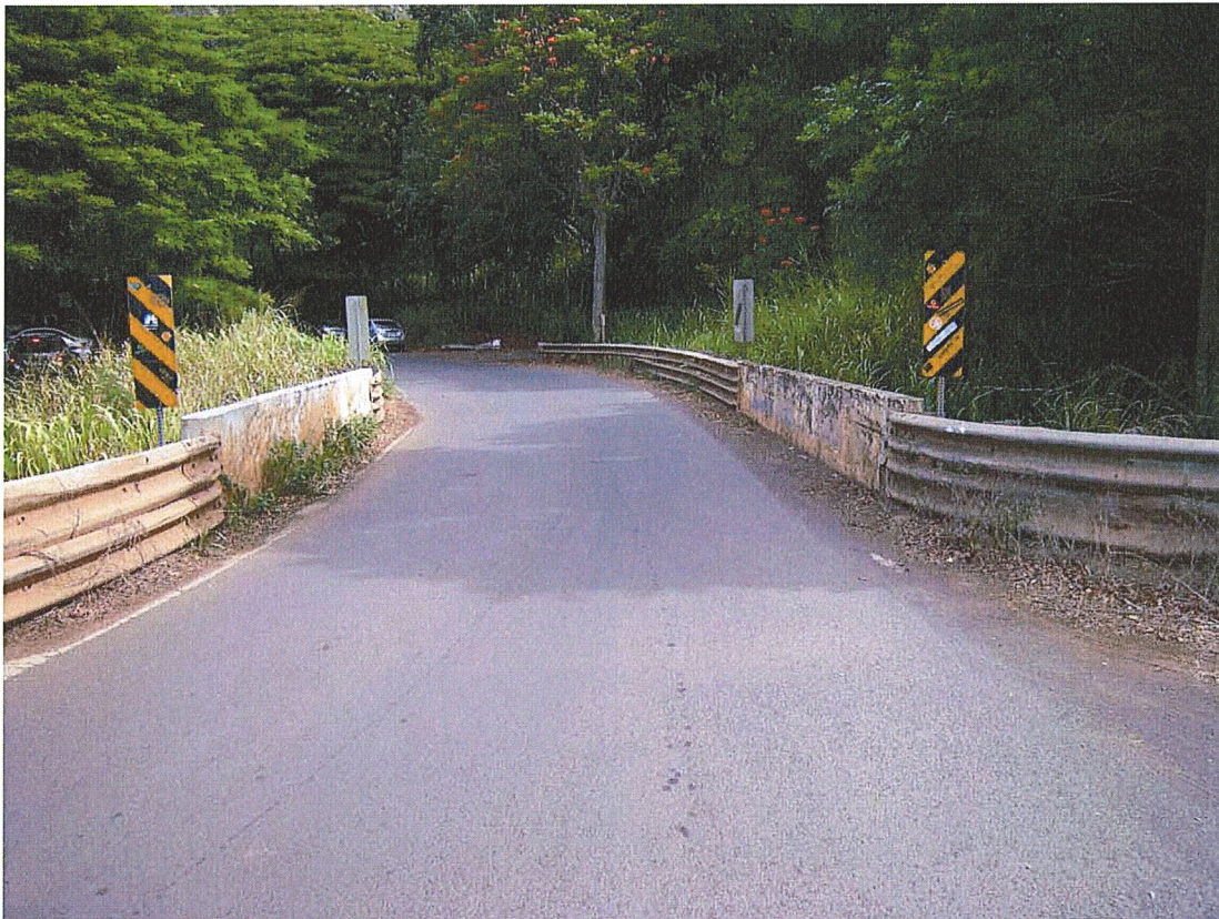
Photograph 1. HI_MauiCounty_HonoluaStreamBridge_0001. Overview of the bridge. View facing north, upstream to the right.
