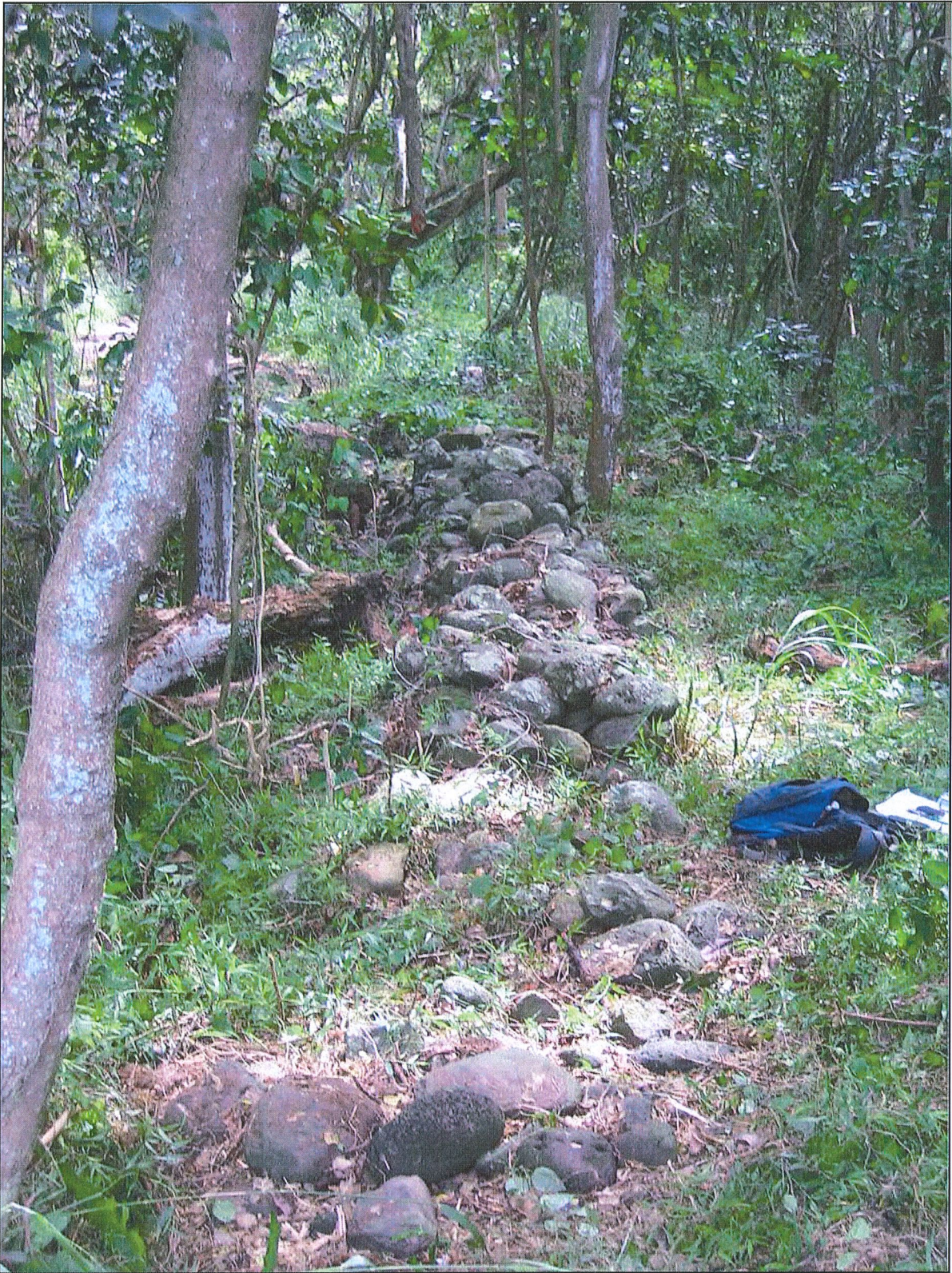
Figure 9: View East of Wall (note collapsed portion in foreground)
