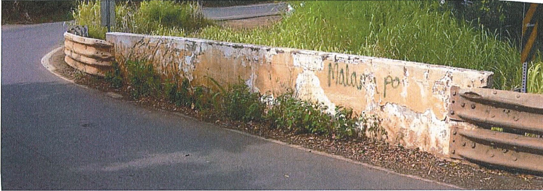
Photograph 5. HI_MauiCounty_HonoluaStreamBridge_0005. Parapet on the downstream side of the bridge. Note the repaired section at the far end. View facing southwest.
