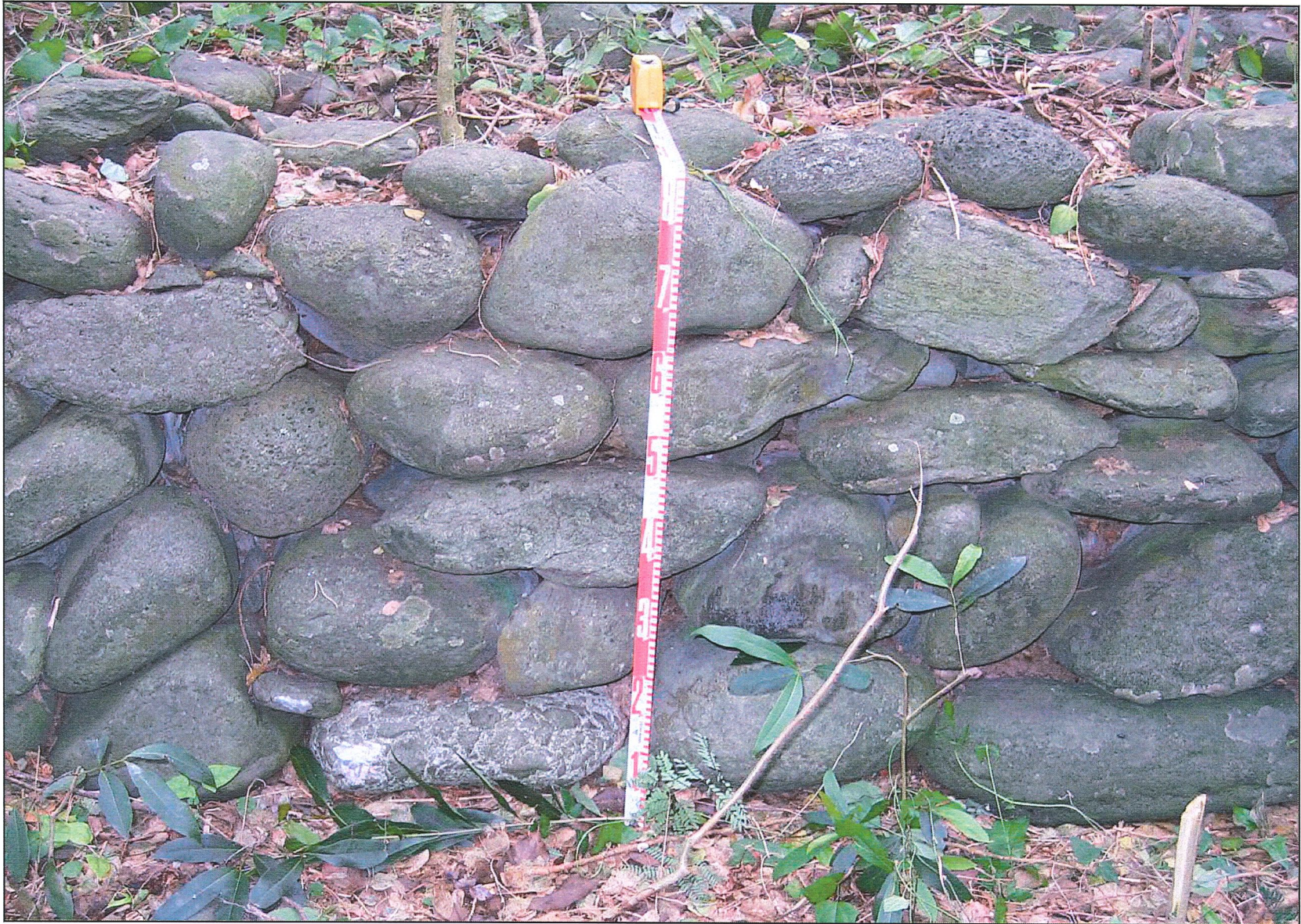
Figure 7: View North of Terrace Wall (note: waterworn aggregate at base on left side of scale tape)
