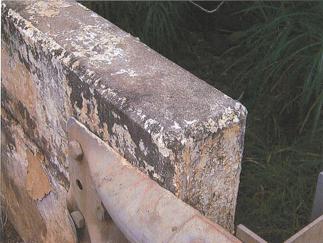
Photograph 8. HI_MauiCounty_HonoluaStreamBridge_0008. Detail of the south end of the upstream parapet showing the chamfered edges. View facing northeast.
