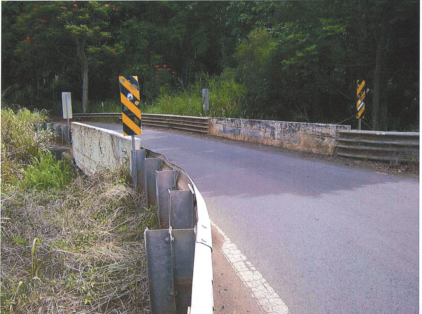
Photograph 2. HI_MauiCounty_HonoluaStreamBridge_0002. Overview of the bridge showing the plain, solid parapets. View facing northeast.
