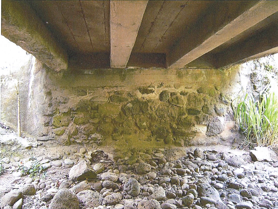
Photograph 11. HI_MauiCounty_HonoluaStreamBridge_0011. Underside of the bridge showing the south abutment. Wood boards fill the spaces between the beams atop the abutment. Note the board formed concrete of the beams and deck. View facing south.
