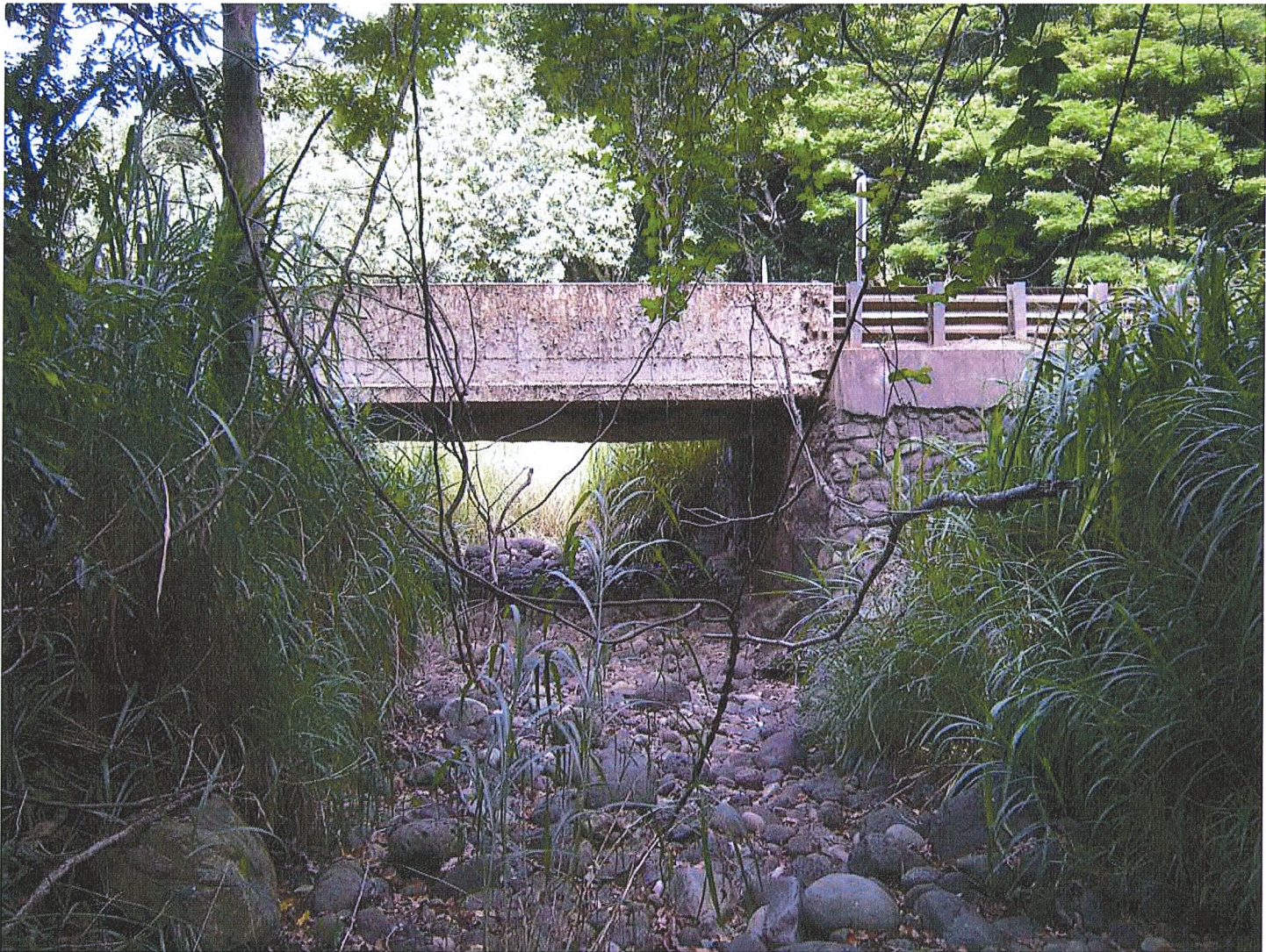
Photograph 4. HI_MauiCounty_HonoluaStreamBridge_0004. View of the bridge from the streambed on the upstream side. View facing west.
