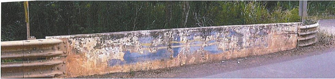
Photograph 6. HI_MauiCounty_HonoluaStreamBridge_0006. Parapet on the upstream side of the bridge. View facing southeast.
