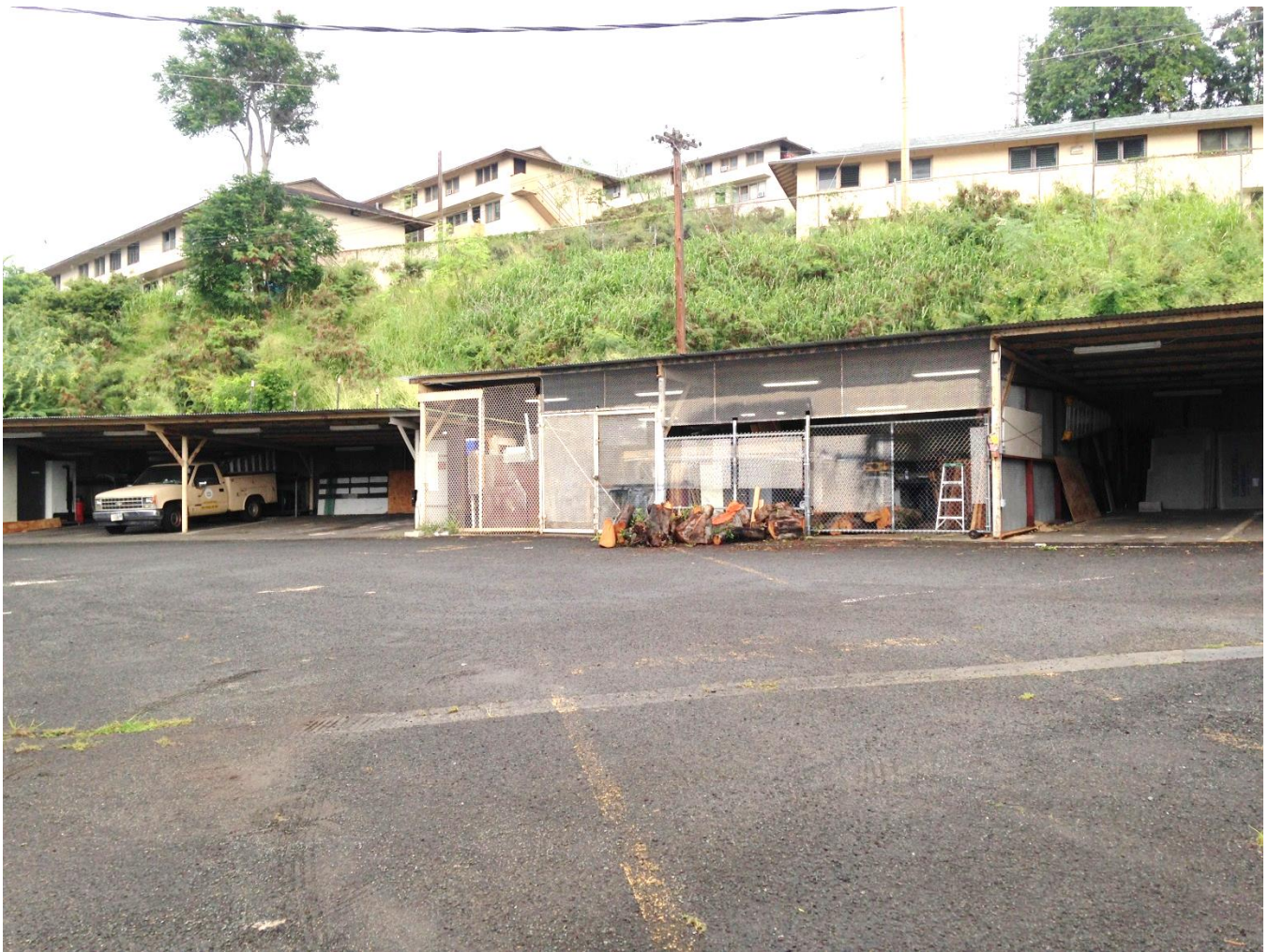
Open, covered garages located at rear of Building D and Central Storeroom.
