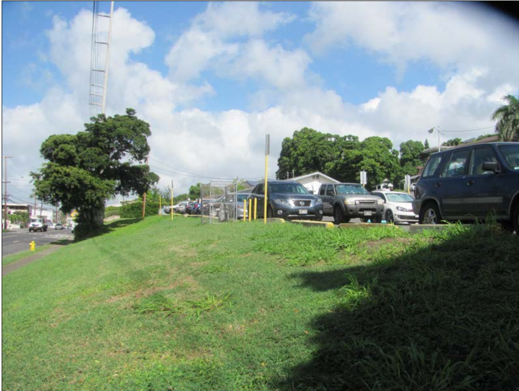
Figure 12. Grading, parking, drainage, utility, and building construction at the northwest end of the study area, view to the north-northwest.
