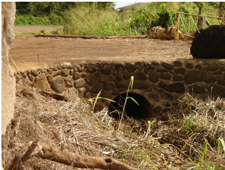
Figure 1: Culvert under a plantation road to Lihue Plantation Mill View to the east toward Kuhio Highway
