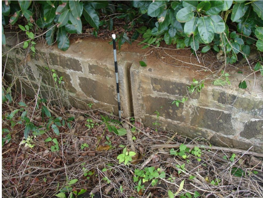
Figure 2: Basalt-lined ditch with slot for water control battens. View to the south
