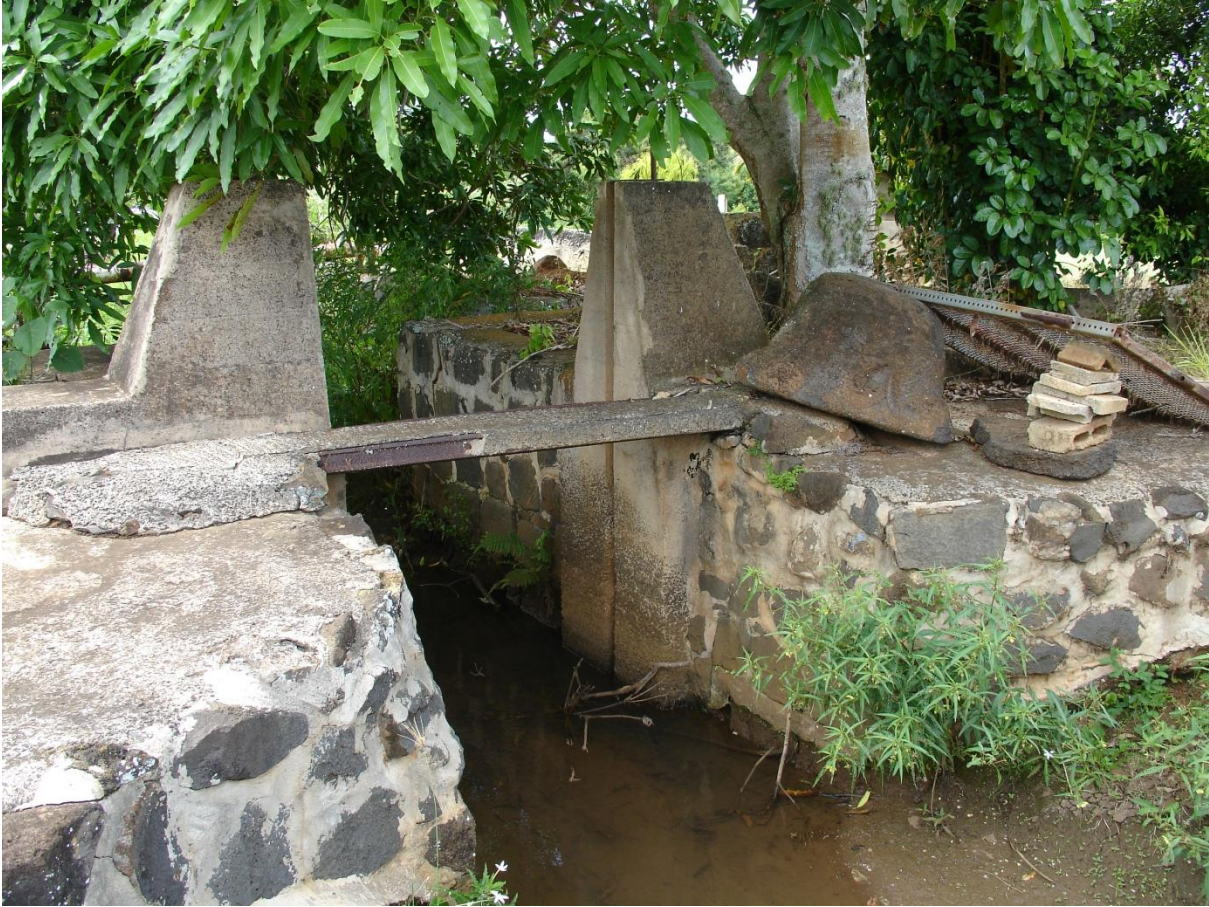
Figure 12: Water control gate for irrigation water from De Mello Reservoir.
