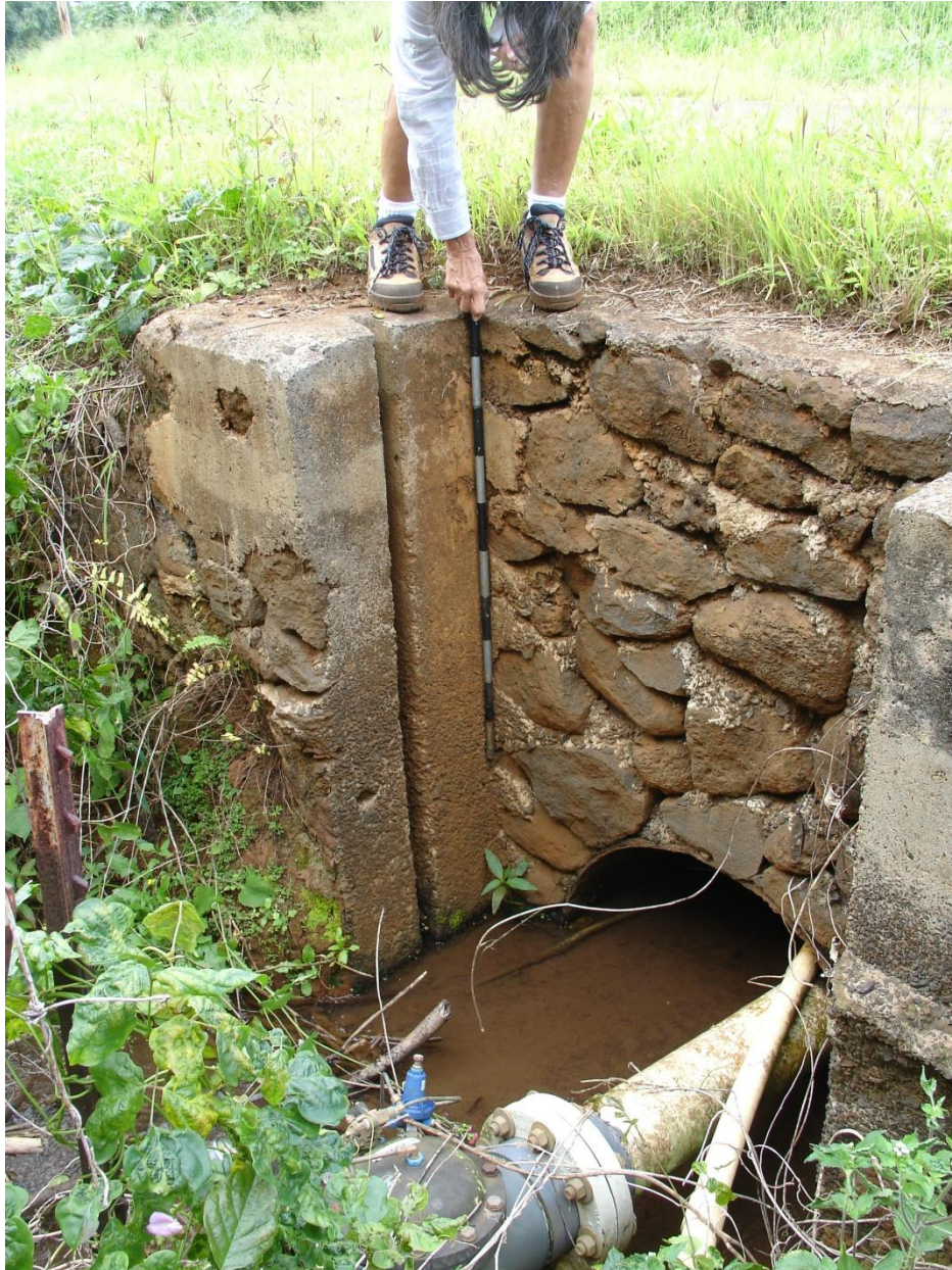
Figure 4: Southside of metal culvert Note plastic pipe system for irrigation water that now directs irrigation water instead of the original open ditch system.
