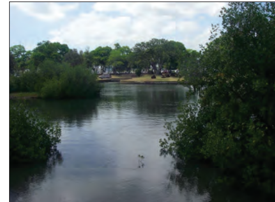
Figure 10. Opening of the culvert that transmits water between the Ala Moana Regional Park system and Kewalo Basin.
