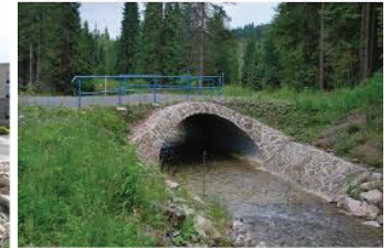
ConSpan Structure – estimated cost $800,000
