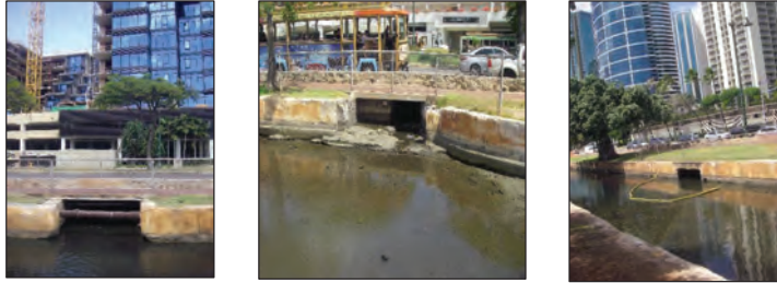
Figure 11. Openings into the canal from culverts passing under Ala Moana Boulevard. Only one has a detritus collector (right).
