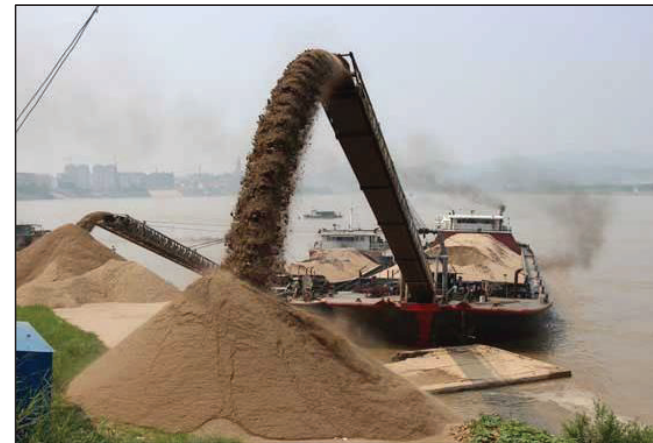
Figure 7-10 Barge-mounted conveyor system
