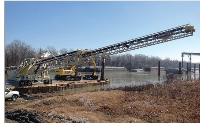
Figure 7-9 Barge-mounted conveyor system
