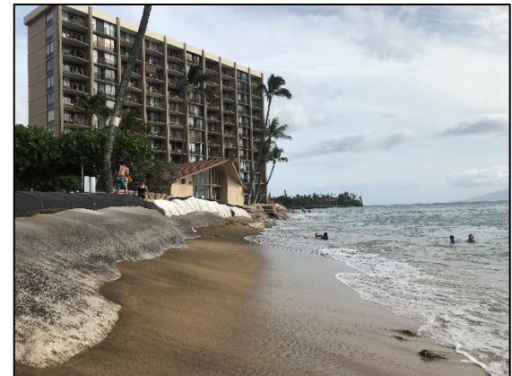
Photo #6 (7/13/18): Looking south at geotextile shoreline protection at Royal Kahana and Valley Isle Resort.
