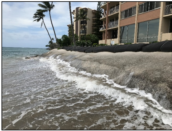
Photo #5 (7/13/18): Looking north at geotextile shoreline protection at Royal Kahana.
