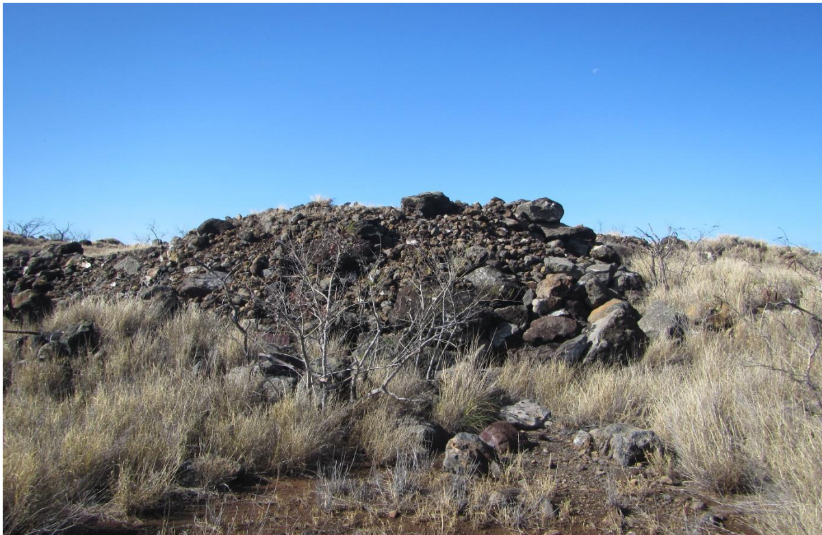
Bulldozer push in NW portion of the project area; view to the northwest.
