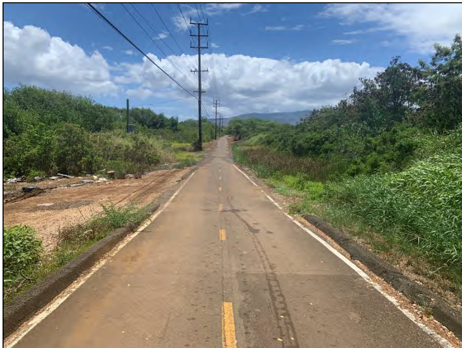
Figure 135. General view of the study area showing the Pearl Harbor Bike Path (OR&L ROW; SIHP # 50-80-12-9714) and peripheral areas within the study area in Waiawa Ahupua'a, view to west
