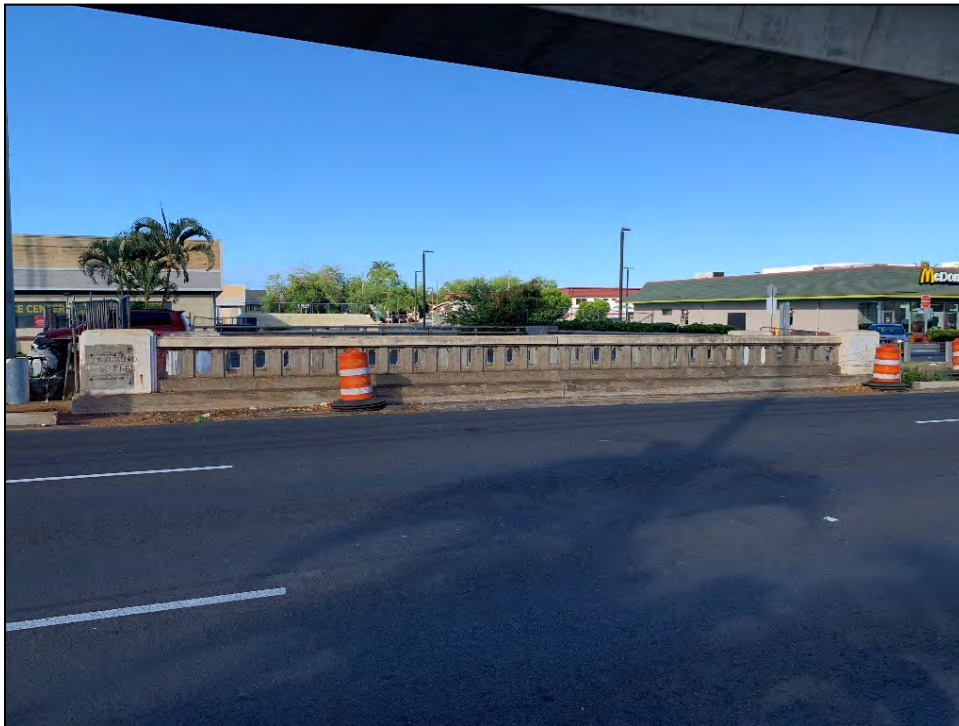
Figure 157. Photograph showing the interior railing of the Kalauao Spring Bridge westbound lane of Kamehameha Highway constructed in 1945, view to southwest
