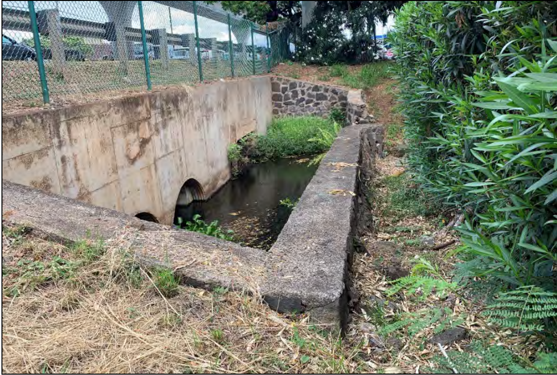
Figure 154. CSH 52, Waiiau Spring weir and culvert on the makai (south) side of Kamehameha Highway, view to northeast
