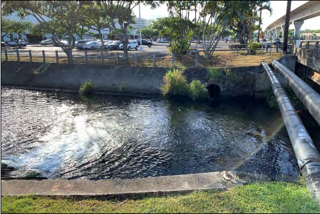
Figure 158. Photograph of Kalauao Spring Bridge and channelized stream below (note two possible channelizing events—mortared basalt, later followed by concrete), view to east
