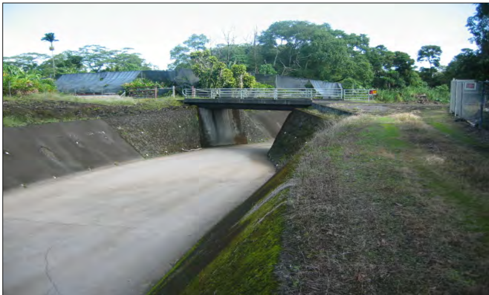
Figure 16. Waiakea Stream looking downstream at the upstream face of the T. Shiroma Bridge (Note channel restriction)
