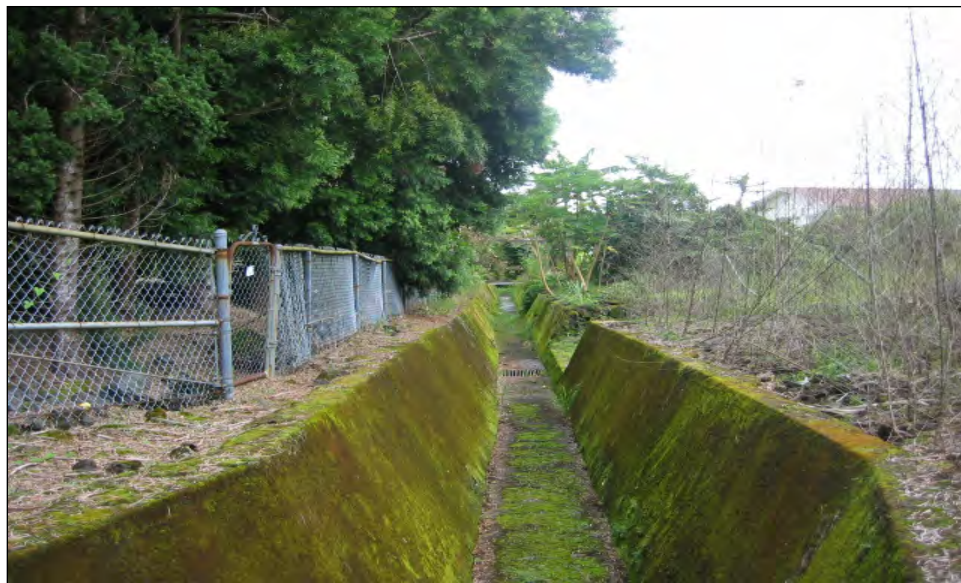
Figure 24. Palai Stream C looking upstream at drainage ditch
