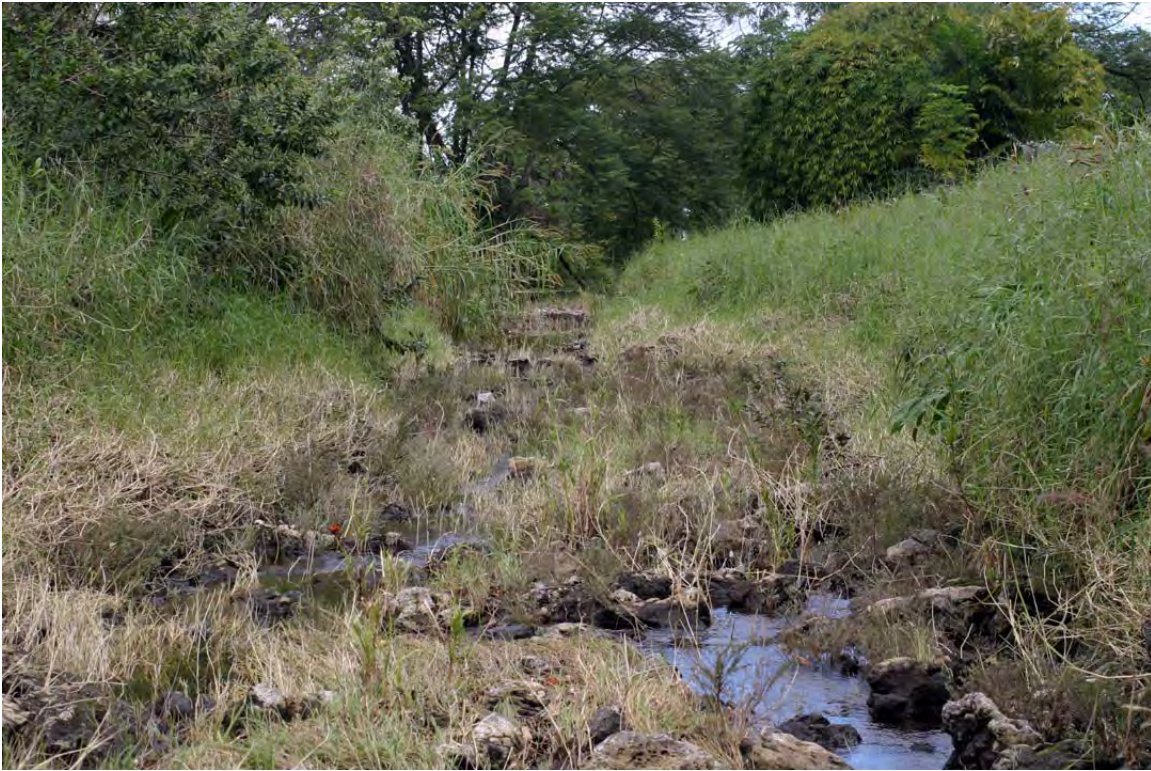
Figure 3. Waiākea Stream above Kupulau Road showing low flow, but evidence (stripped and bent grass) of much stronger flow sometime prior to December 8, 2009. Vegetation here is mostly para or California grass.
