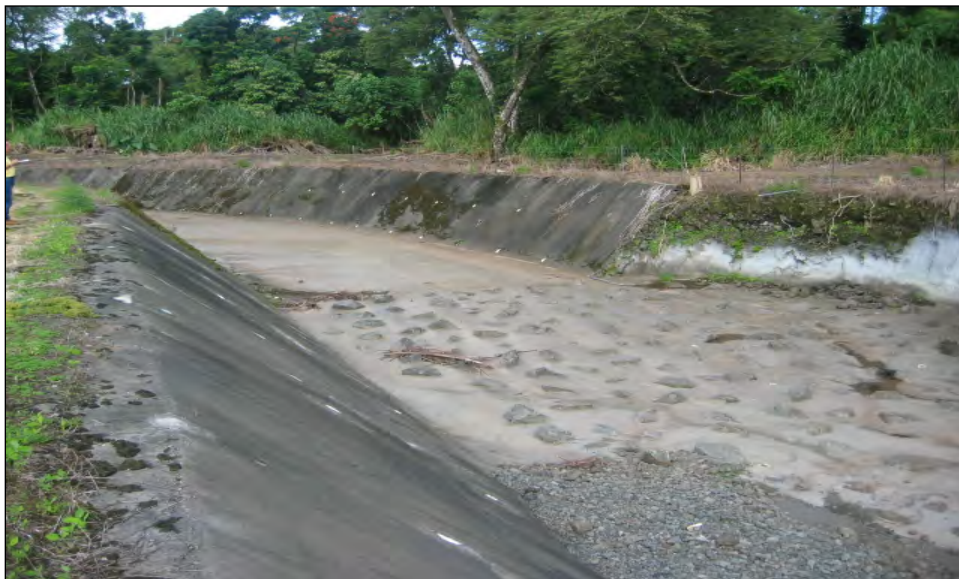
Figure 18. Waiakea Stream looking upstream at Waiakea-Uka channel from Station 18+00 Note scour damage repair on right bank.
