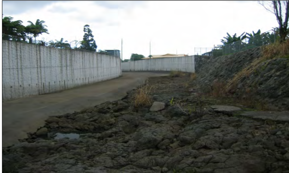
Figure 11. Waiakea Stream looking downstream from the end of the channel lining towards Kawailani St
