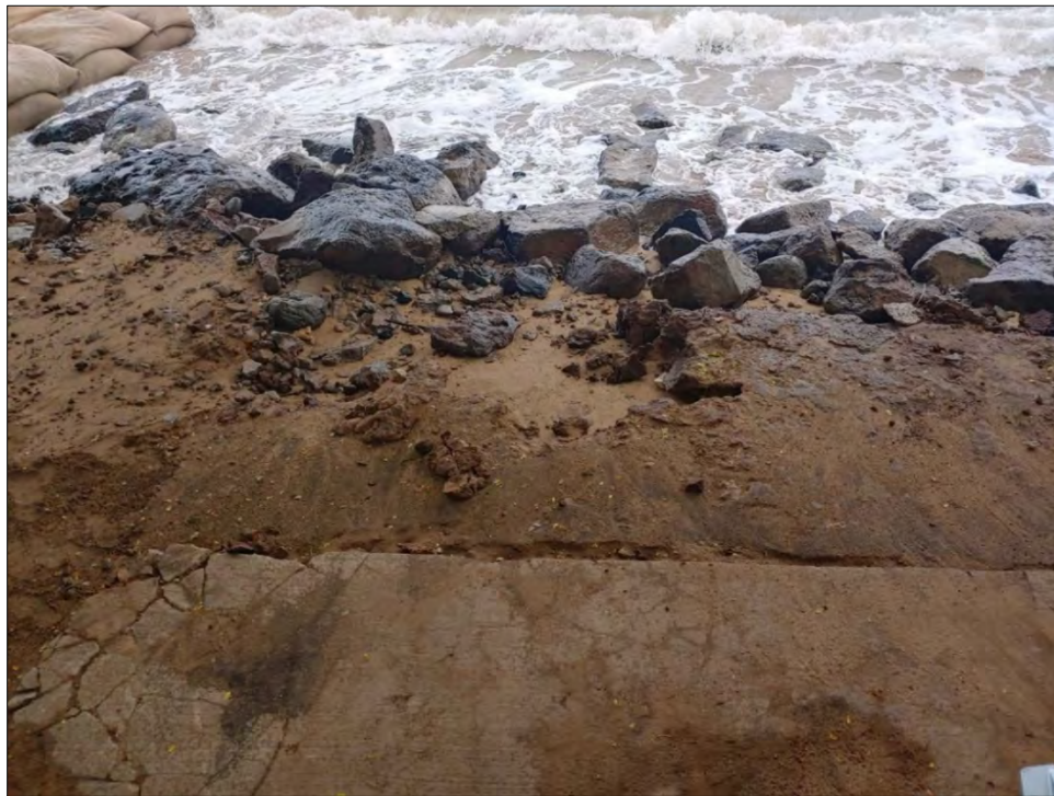
Figure 43. Coastal erosion at the Sadang property (Courtesy of Mr. Felimon Sadang)
