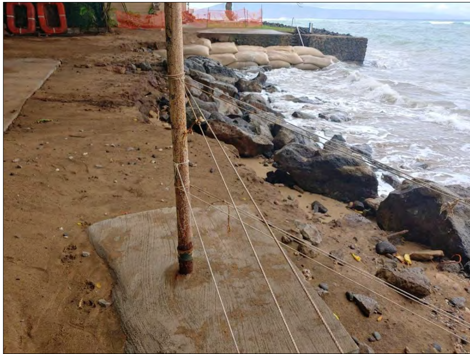
Figure 41. Coastal erosion at the Sadang property. Compare this to Figure 7. Cement foundation gone and sandy area fronting the property (Courtesy of Mr. Felimon Sadang)
