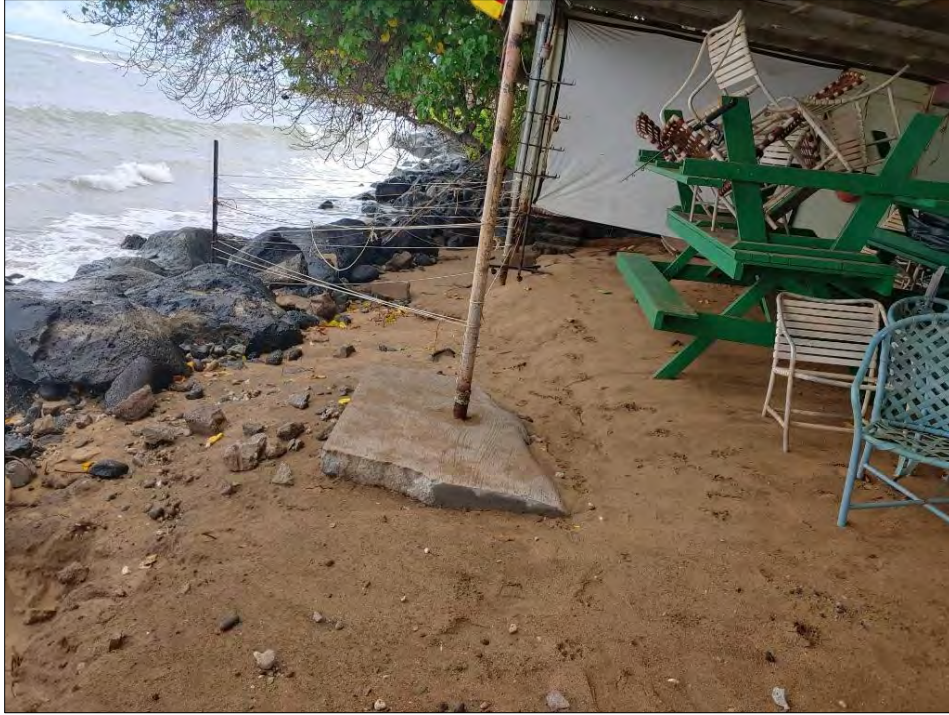
Figure 40. Coastal erosion at the Sadang property (Courtesy of Mr. Felimon Sadang)
