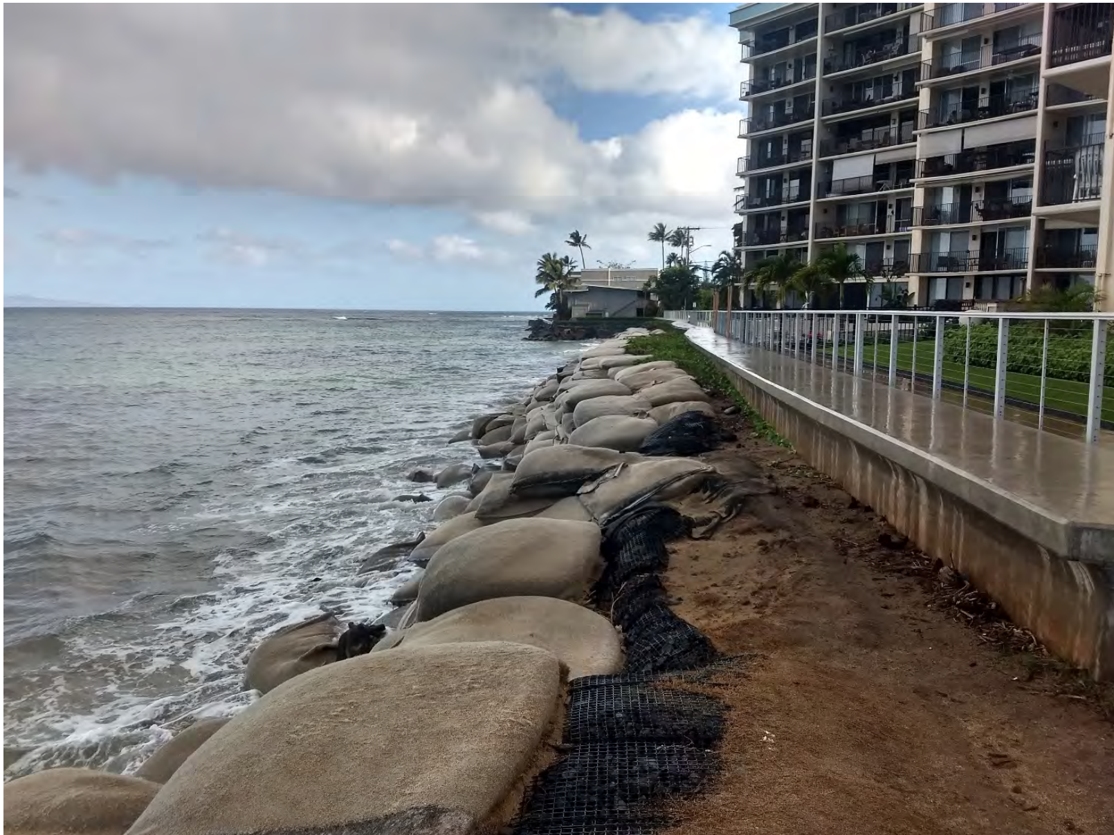
Figure 11: Coastal Photographic View of a Seaward Facing Portion of the Hololani Resort and Sandbags Along the Shoreline. View to the North.
