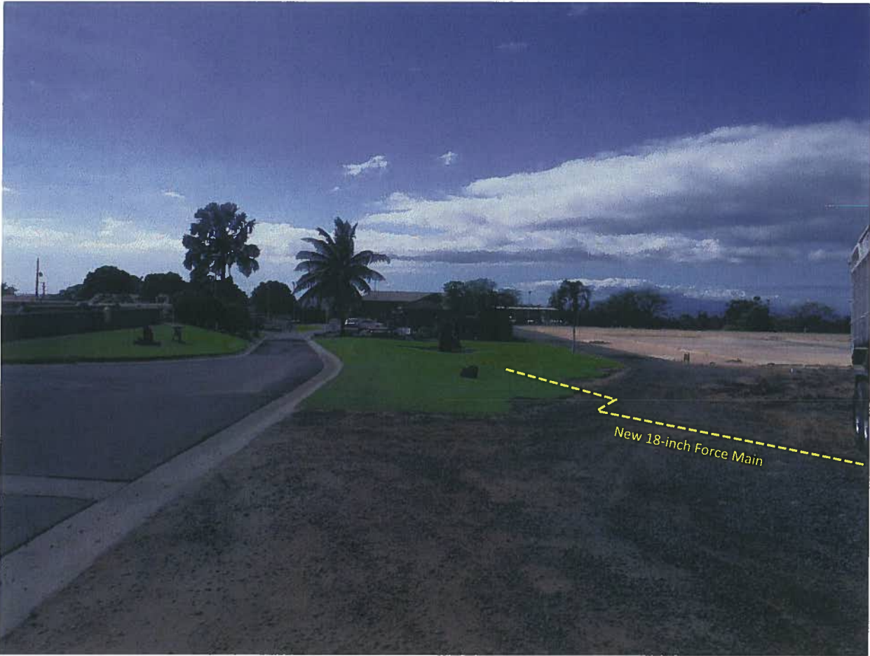
Photo 3: Existing Kihei Wastewater Reclamation Facility (WWRF); general location of new 18-inch recycled water line.
