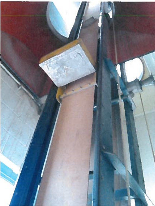
Conveyor belt elevator System from 1 st to 5 th floor
