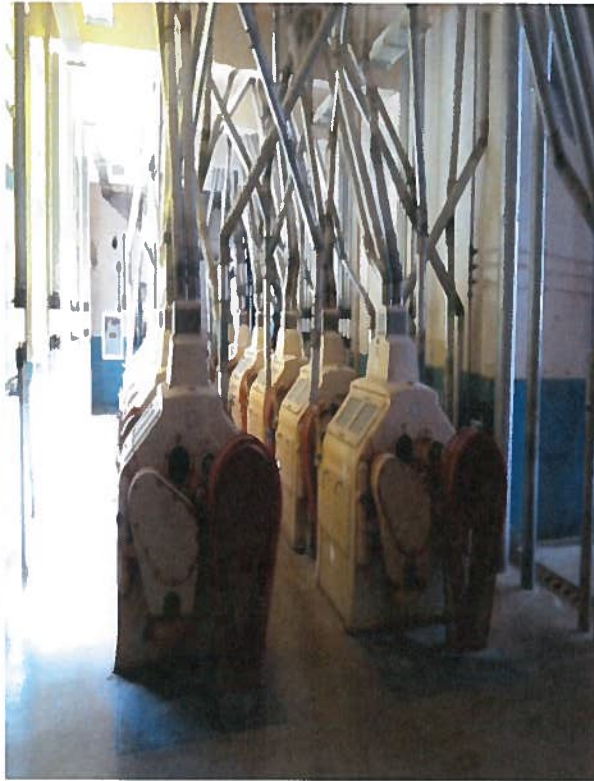
Elaborate pneumatic tube system 1 st to 5 th flr.
