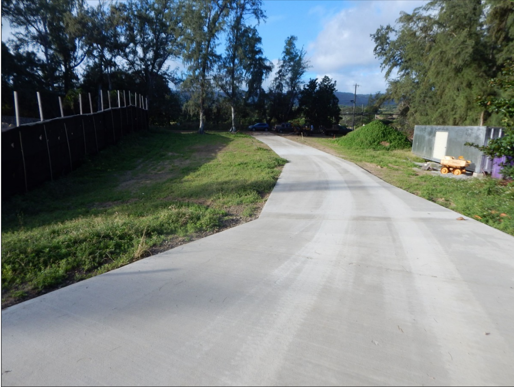
Figure 7. Concrete driveway extending through the center of the Tax Map parcel, view to the southwest.
