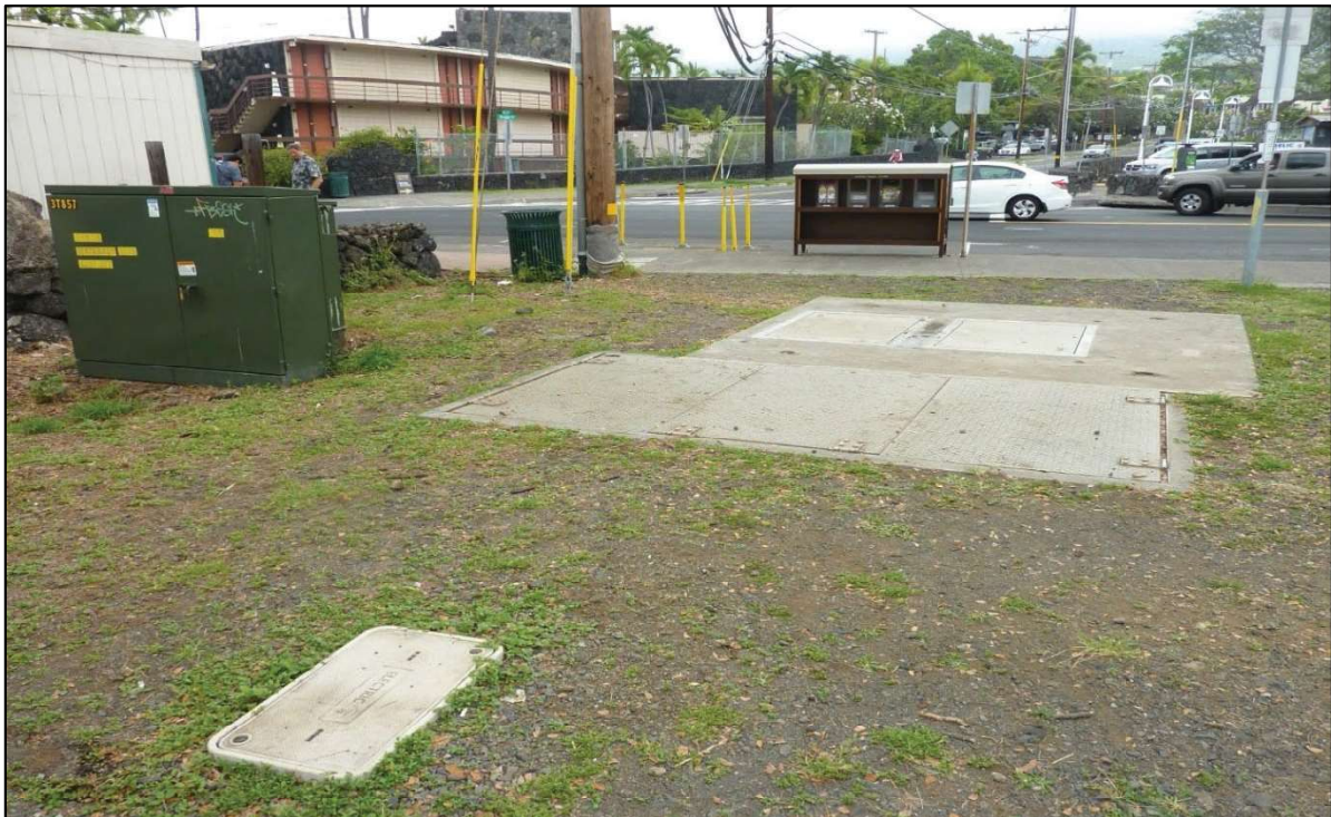
Photo 2. Alternate view of sewer pump station looking mauka, towards Hualalai Road.
