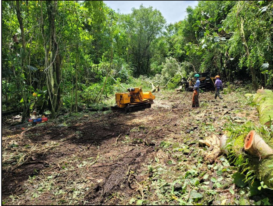
Figure 22. Photo of Tree Works crew clearing vegetation along a portion of the existing force main corridor within the project area; view to southwest
