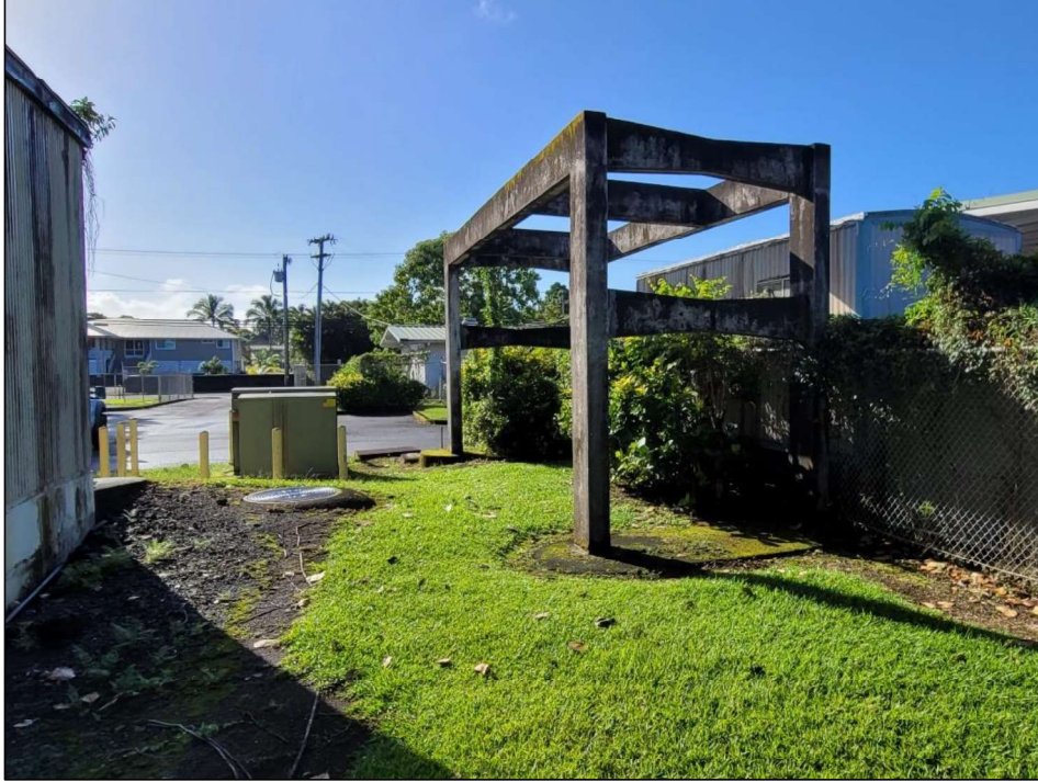
Figure 41. Photo showing the concrete structure located west of the pump station and operations building at the Pua SPS facility; view to south
