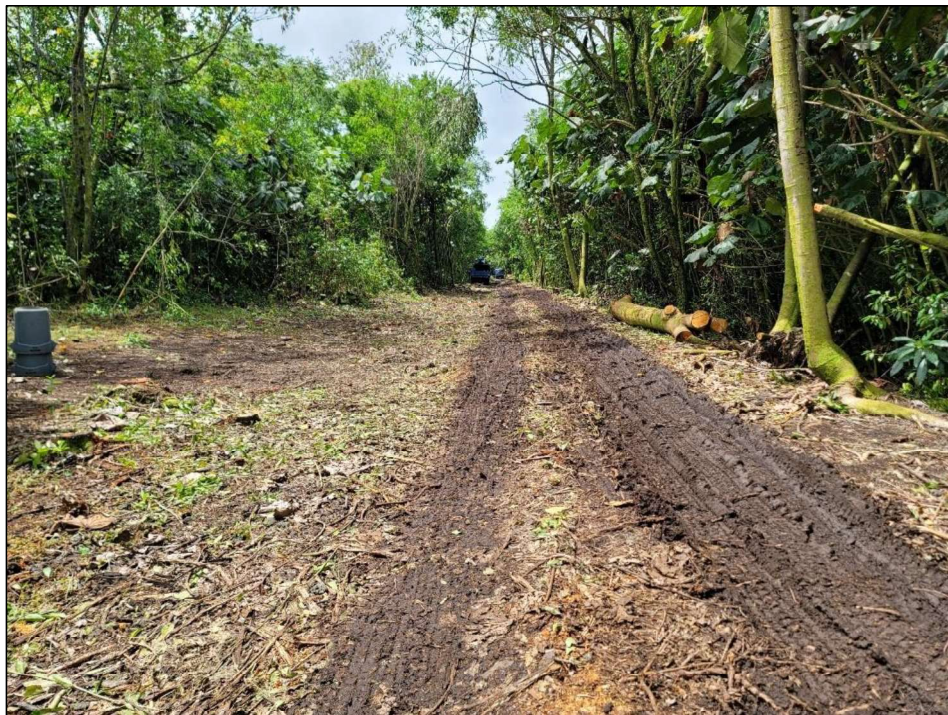
Figure 23. Photo overlooking a recently cleared portion of the existing force main corridor within the project area; view to south
