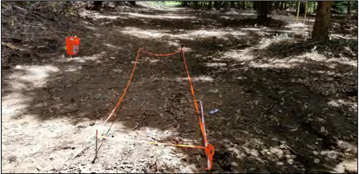
Figure 47. Photo of TE 2 marked out with flagging tape prior to excavation; view to southeast
