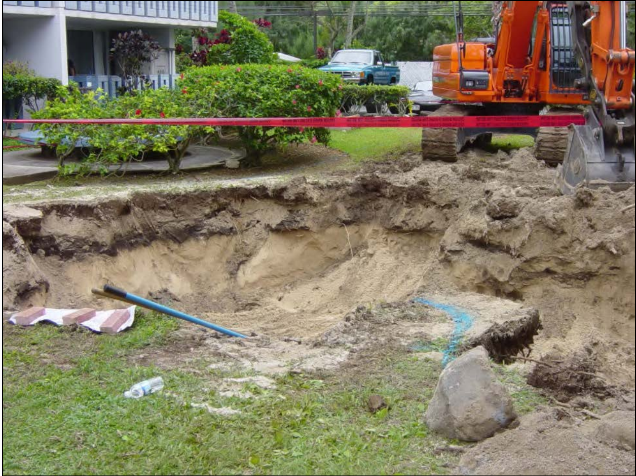
Figure 7: Photographic Overview of Extensive Leach Field Excavation in Progress. View to South.
