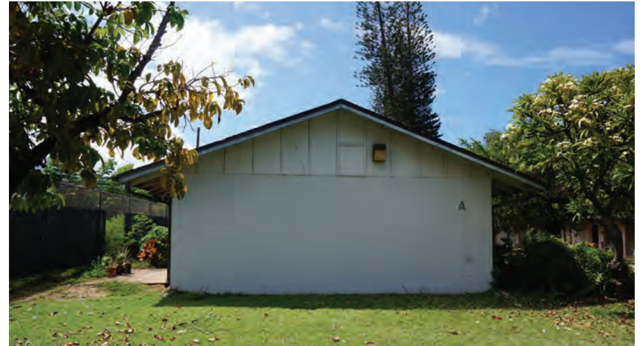
Figure 135: Piilani Homes Building A Left Elevation (right side similar) Source: Fung Associates Inc., 2020
