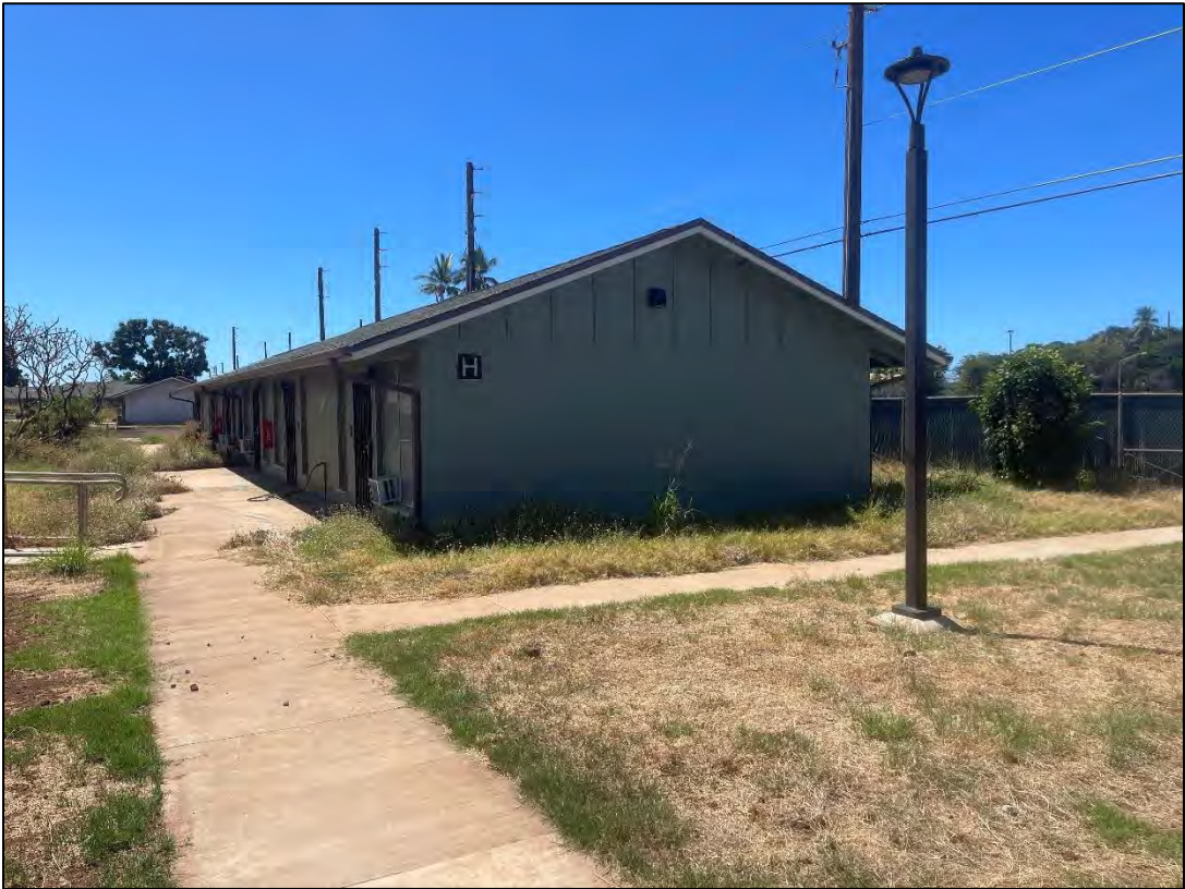
Figure 5. Southwest facade of Building A (above) and northwest and northeast facades of Building H (below). (MASON, September 2024)
