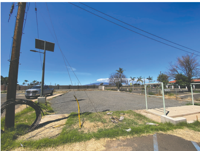
Photo 5 (facing southwest): View of remaining utility structures at northwestern end of David Malo Circle.
