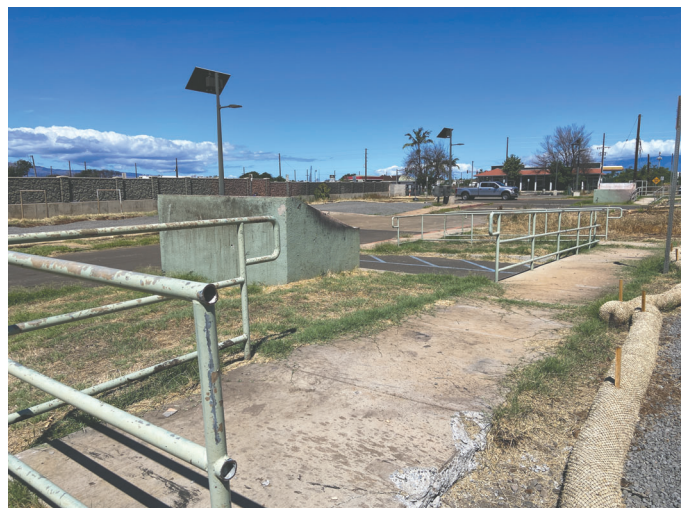
Photo 6 (facing west): View of remaining utility structures at center of David Malo Circle.
