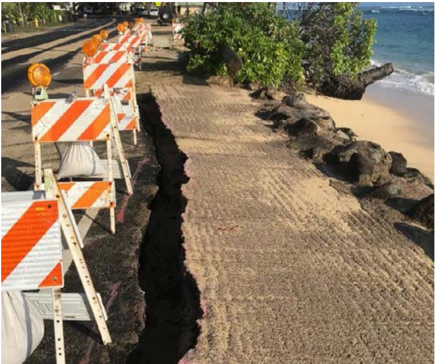
Shoreline erosion in Ka'a'awa, on the windward side of O'ahu, requires the stabilization of adjacent and critical Kamehameha Highway
