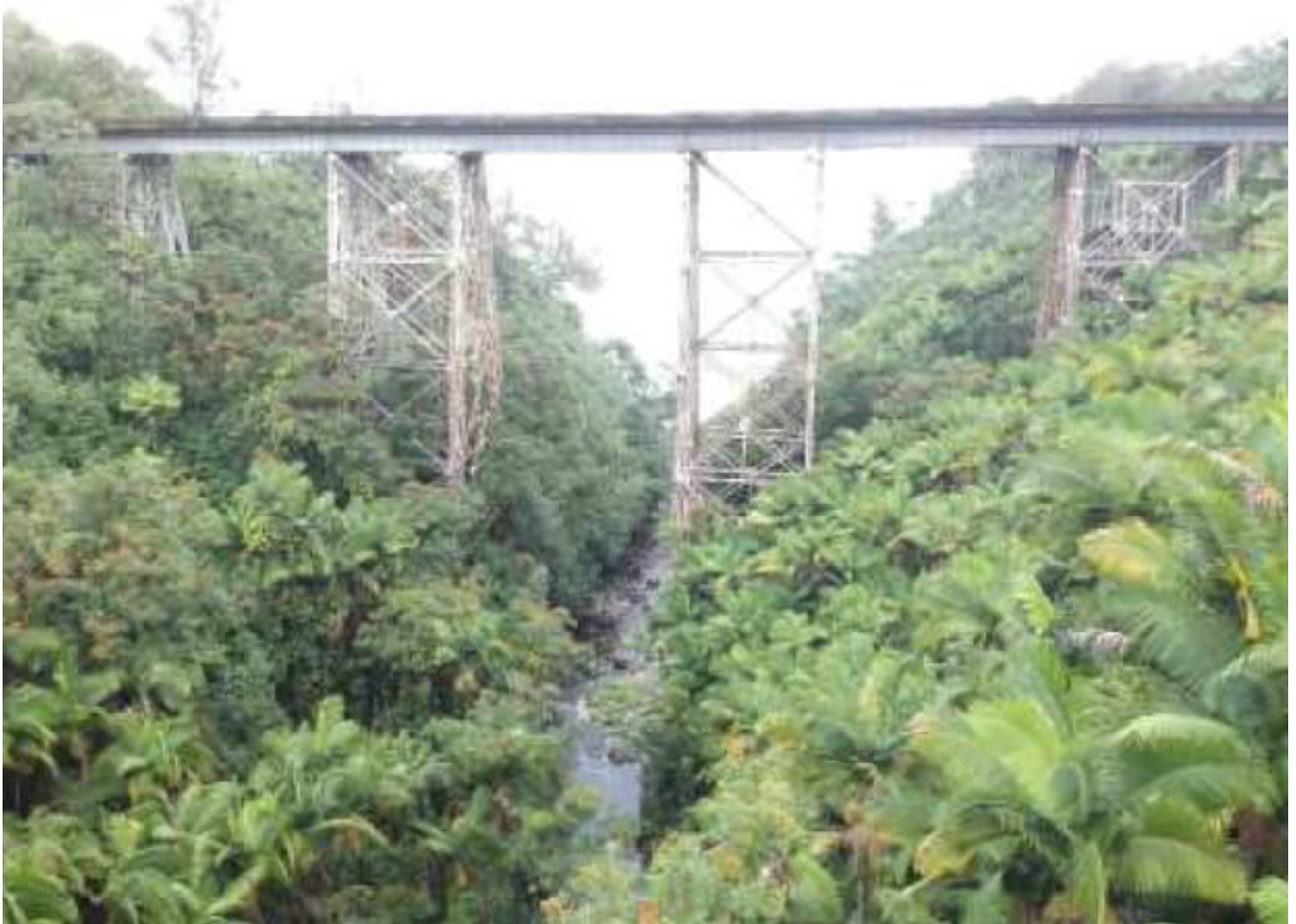
The historic Nanue Stream Bridge along the Hamakua coast of the Big Island is proposed for rehabilitation
